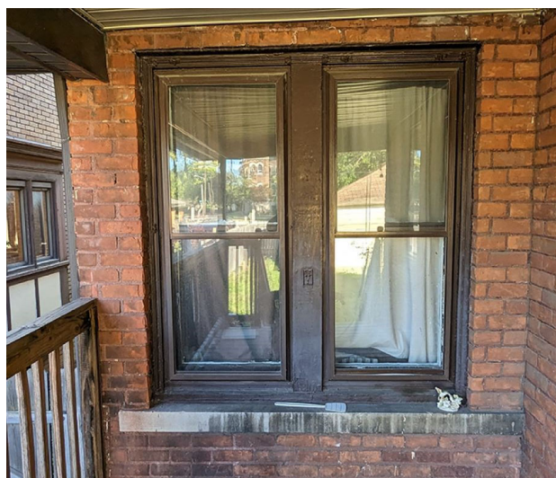
Site Photo 5, by applicant showing original pair of double-hung windows and mullion proposed to be replaced by casements.
