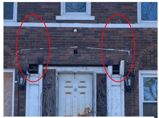
Photo 6, by staff November 28, 2023: front elevation detail showing hints of a Juliette balcony railing over the entrance façade, indicated inside the red circles.
