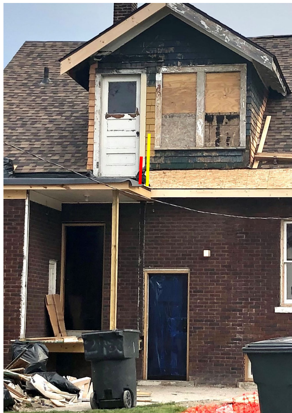
Staff photo, October 25, 2023. The red line identifies the height of the historic knee wall. The yellow line identifies the height of the proposed wood railing.
