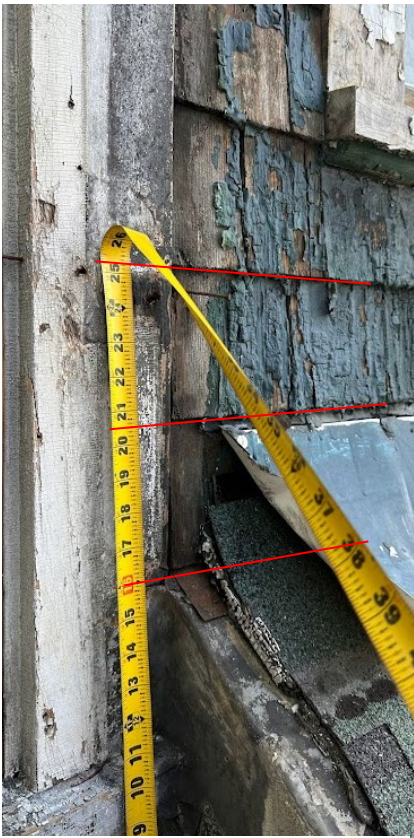
Applicant photo. The exposure of one row of shingles is 4-1/2 inches.
