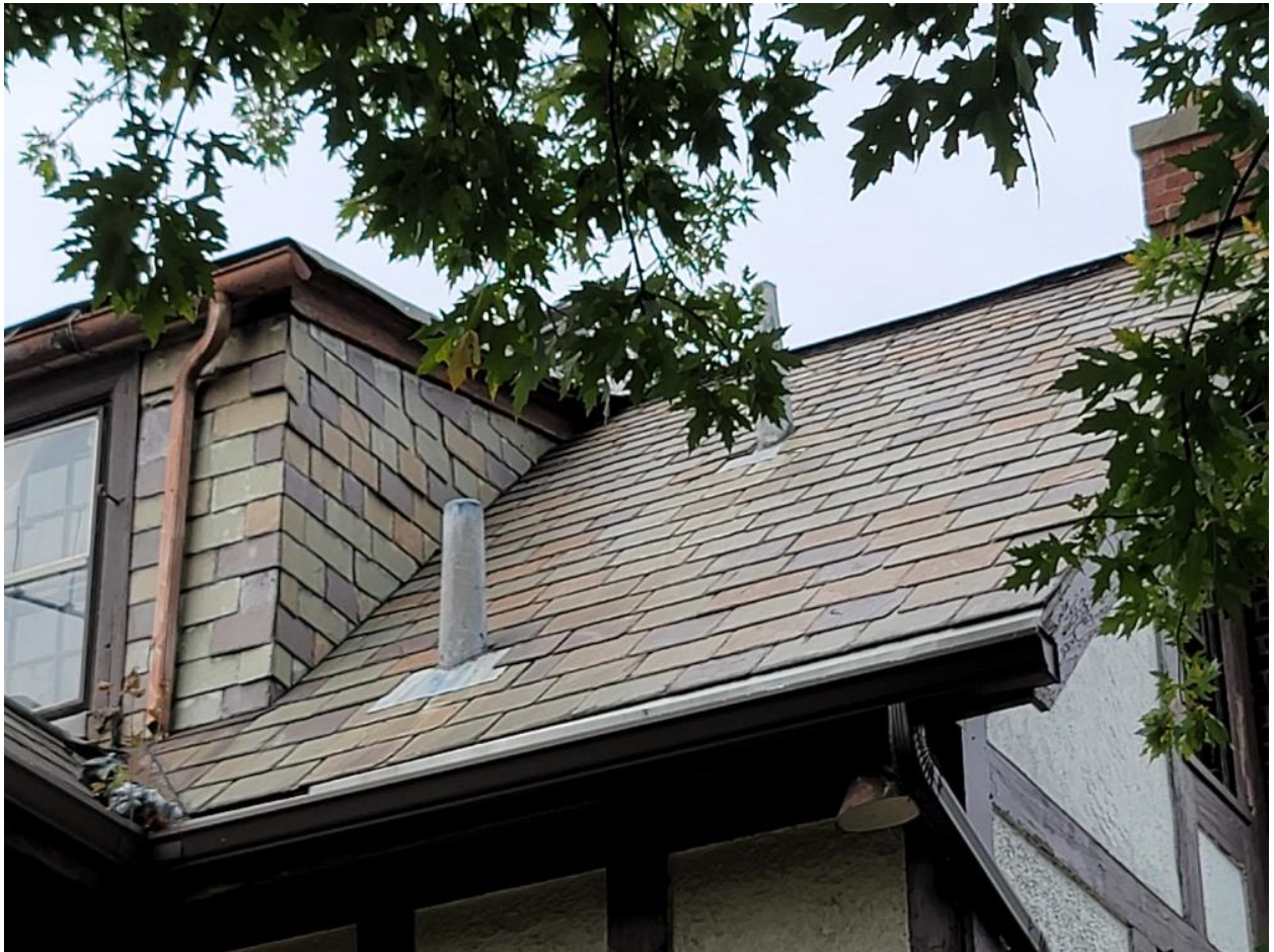
Rear gabled wing and dormer, showing current conditions, facing northwest. Photo taken by applicant
