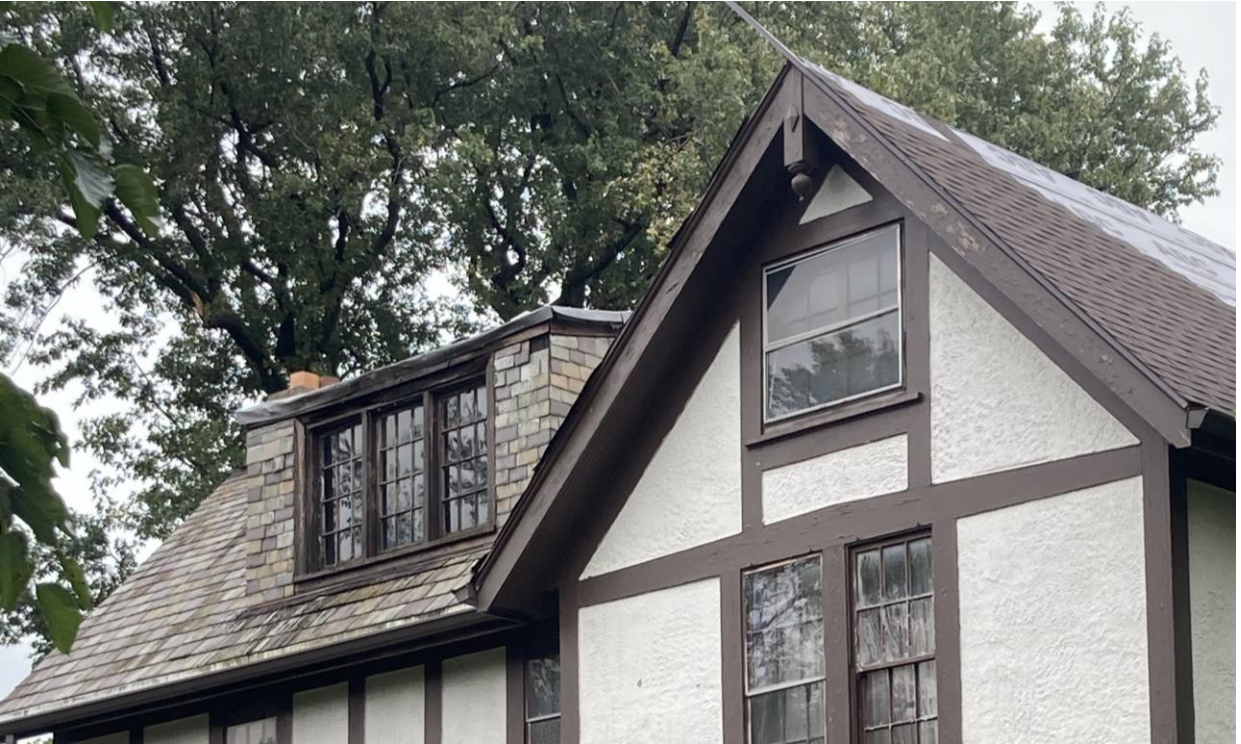
Rear gabled wing and dormer, showing current conditions, facing southeast. Photo taken on 11/1/2023 by staff
