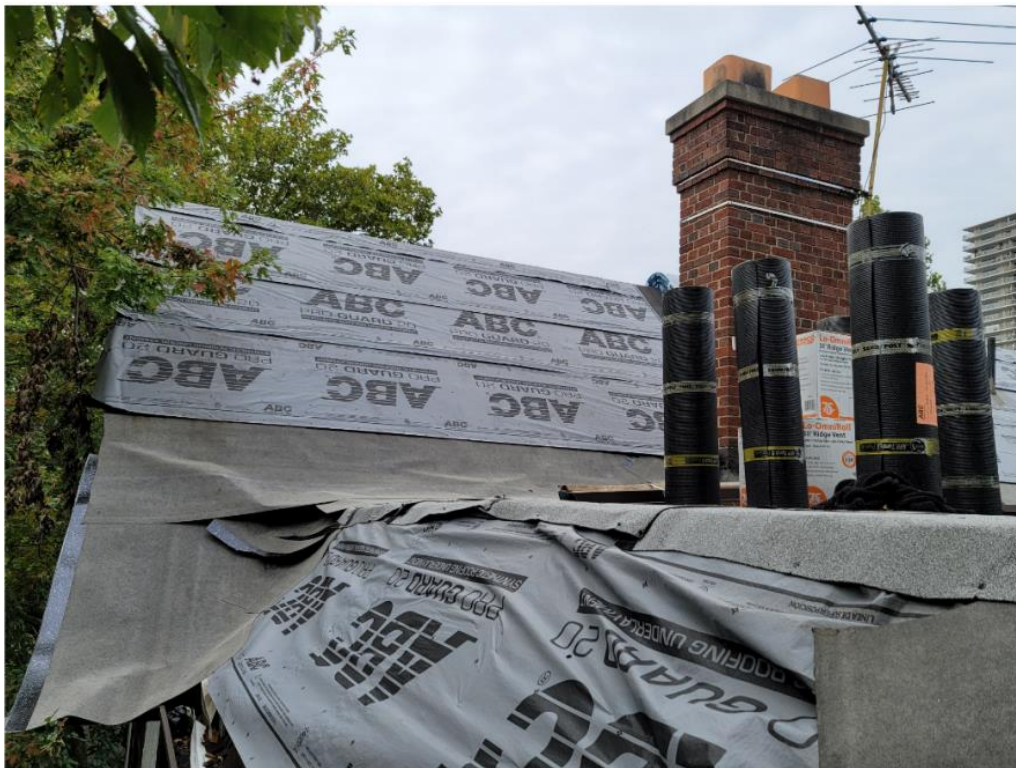
Rear of main side-gabled roof, south portion, facing northwest. Current conditions. Note that the slate has been removed and the area has been covered/weatherproofed with underlayment. Photo provided by applicant
