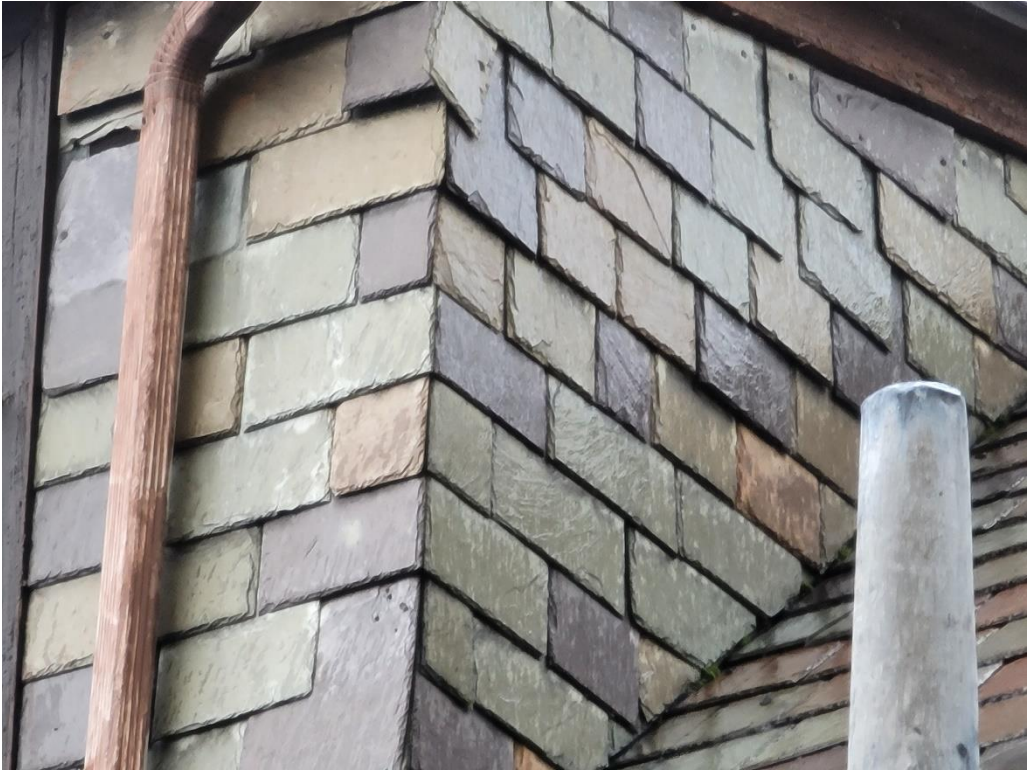
Detailed photos of the remaining slate at the rear roof and dormers, provided by applicant
