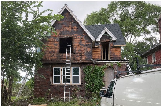
Site Photo 3, by Staff July 21, 2023: (West) front elevation, showing work in progress without approval.
