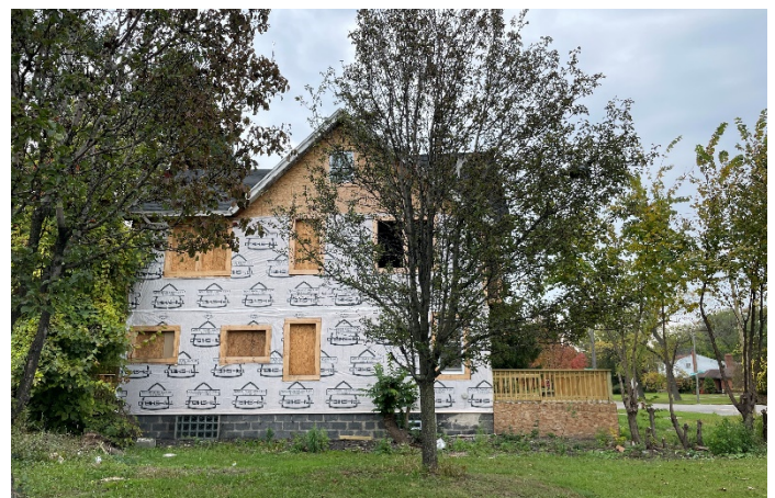
Site Photo 4, by Staff October 19, 2023: (North) Side elevation showing removed windows, removed brick and shake siding, and installation of the front deck.
