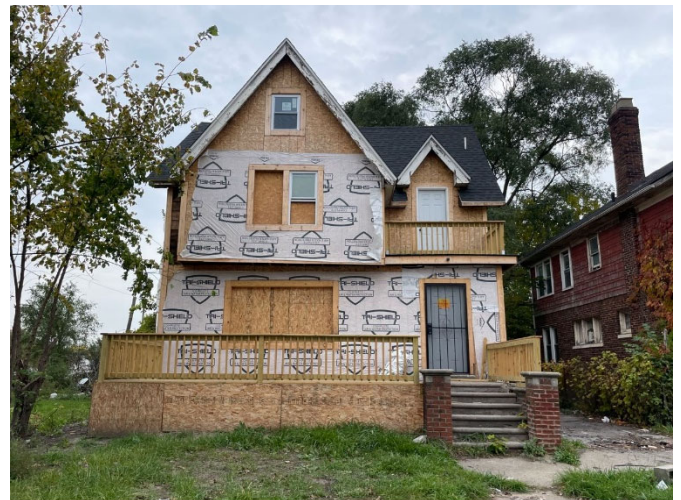
Site Photo 1, by Staff October 19, 2023: (West) Front elevation showing replaced roof, removed chimney, removed arched doorway, bay windows, siding, porch, and other features, and introducing new window in the gable without approval.
