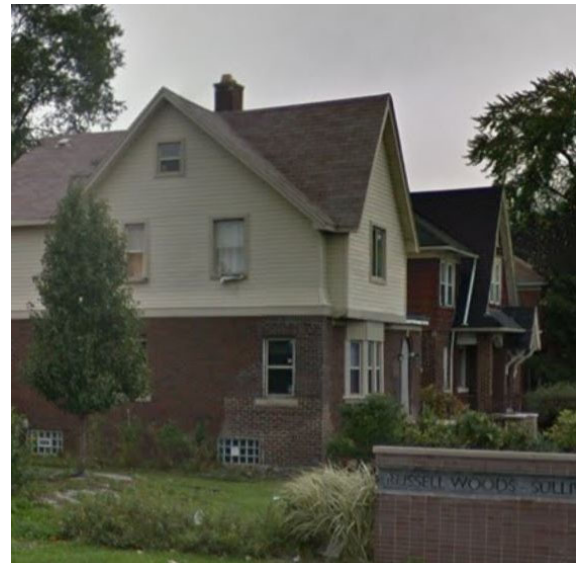
Site Photo 6, by Google Streetview October 2011, showing shake siding covered with vinyl, brick wall extension removed and patched with new mortar.
