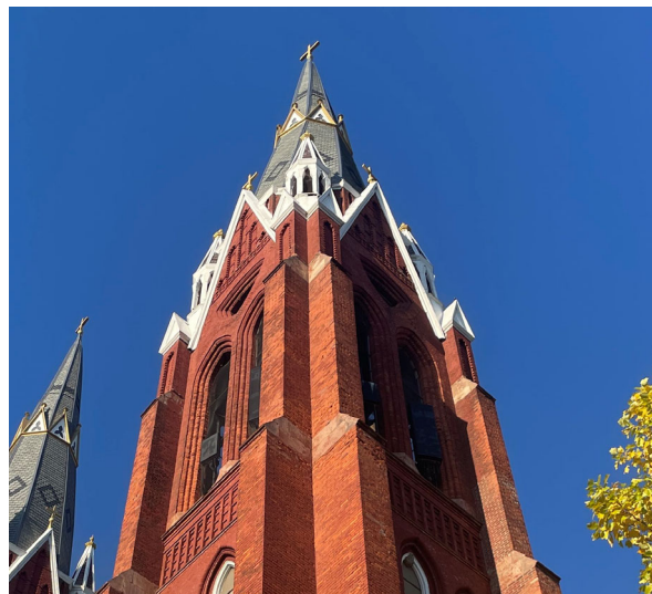
Site Photo 2, by Staff October 24, 2023: Southwest side of south tower showing currently installed telecommunications equipment outside the tower windows. The west face (left) is the proposed installation, the south face (right) is the equipment under violation.
