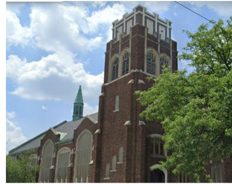
Site Photo 6, by Google Street View 2022: (Northeast) front side of Faith Church (897 Philip St.), showing antennae installation inside new enclosure on tower.
