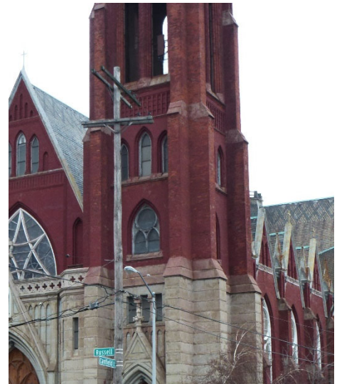
Site Photo 4, by Staff January 24, 2012: (West) front side, showing older antennae installation.
