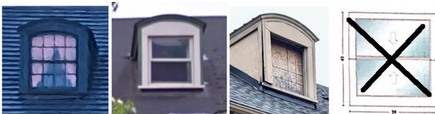
North-facing dormers, left to right: 1980 (Historic Designation Advisory Board), 2007 (Google Maps), existing condition (photo by staff), proposed replacement (from submitted window schedule).
