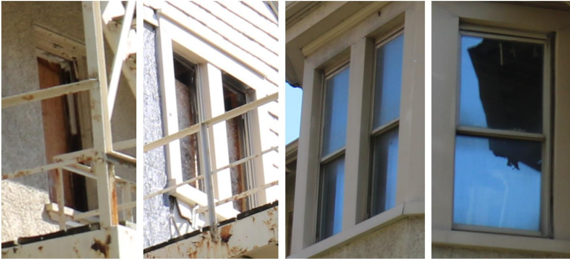
Examples of missing windows and vinyl windows on the property. October 2023 photos by staff.
