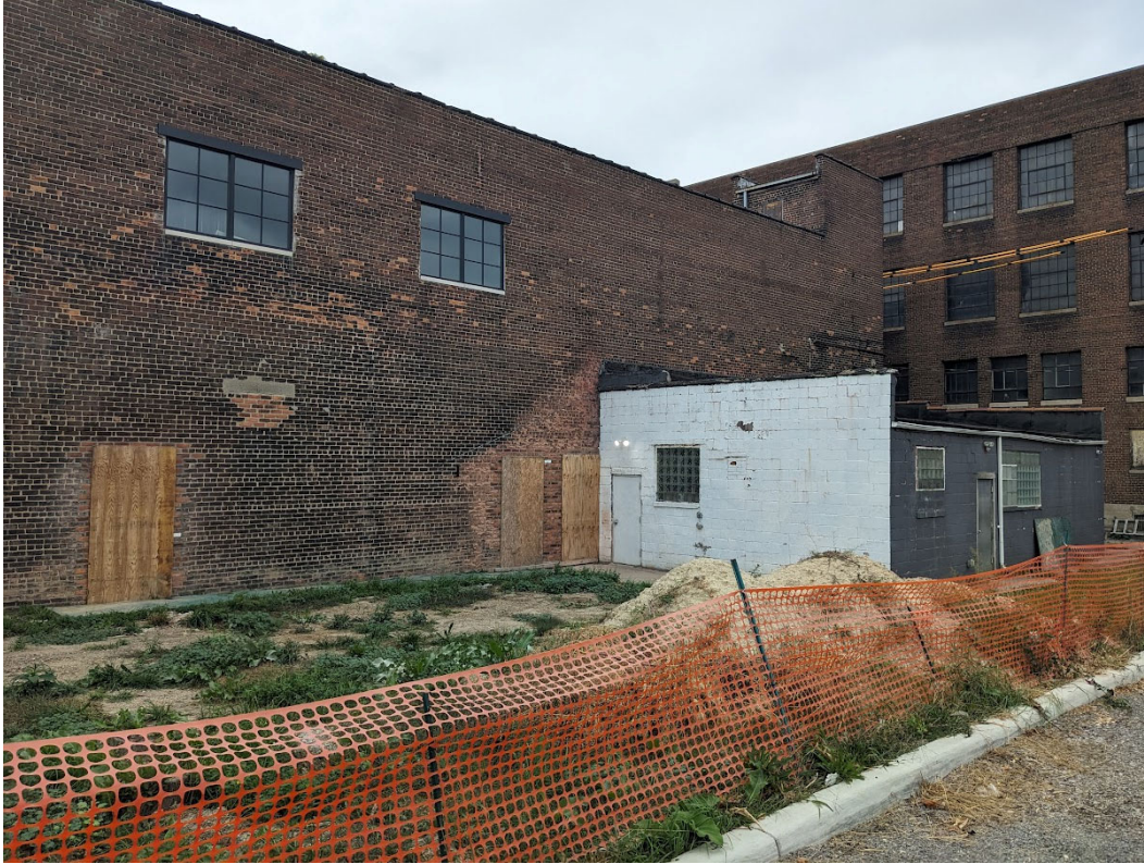
Existing concrete block addition at side of building. Note new entrances being constructed. This existing addition has already been approved for demolition by the Commission; the new structure is proposed to be built in the same general location. View to the northwest from East Milwaukee. Staff photo, September 27, 2023.
