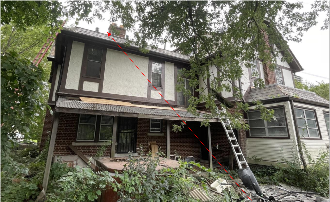
400 Fiske, current appearance of rear wall/roof. Staff photo taken 9/8/2023. Note that a new rubberized roof membrane is proposed for installation at the flat portion of the mansard roof at this location.
