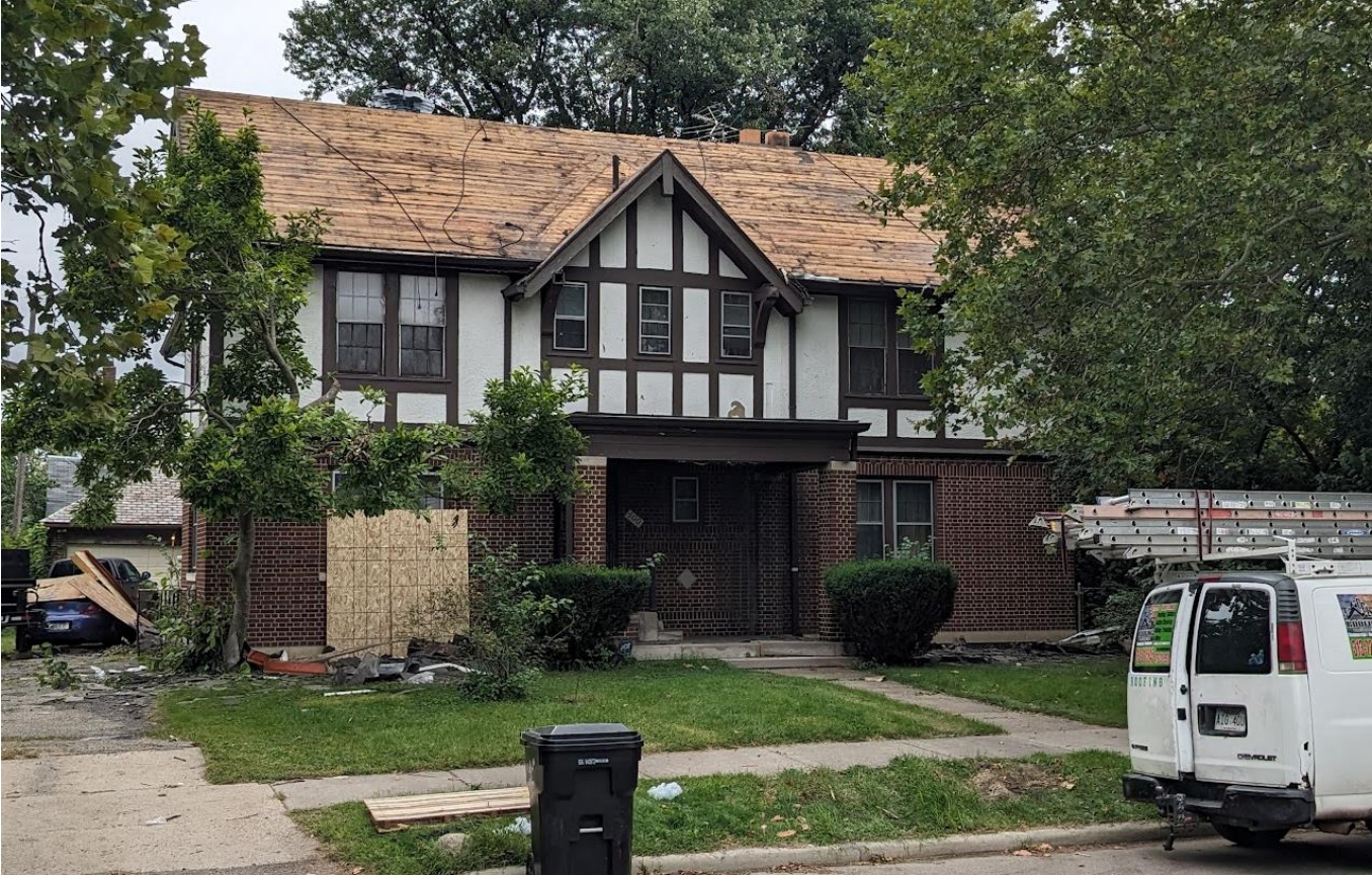
Staff photos, taken on 9/8/2023 during unapproved slate roof removal
