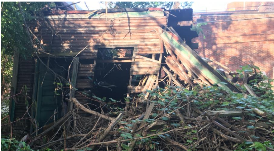
2018 photo of the collapsed garage, provided by the applicant.
