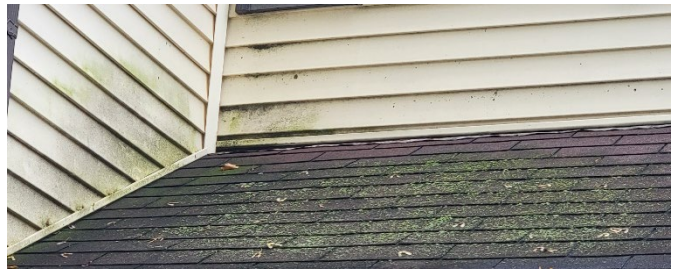
Site Photo 5, by Applicant: (East) front elevation, showing roof condition.
