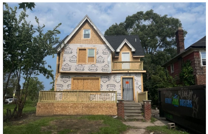
Site Photo 3, by Staff August 24, 2023: (West) Front elevation showing replaced roof, removed chimney, removed arched doorway, bay windows, siding, porch, and other features, and introducing new window in the gable without approval.
