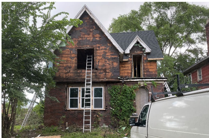
Site Photo 2, by Staff July 21, 2023: (West) front elevation, showing work in progress without approval.
