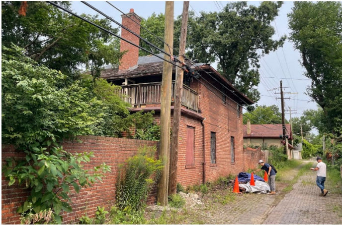
Site Photo 4, by Staff, August 1, 2023: Southeast elevation of carriage house, showing removed roof materials and balcony railing.
