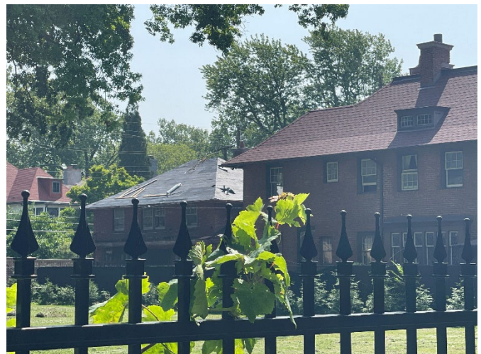
Site Photo 2, by Staff August 3, 2023: (North) side elevation of house and carriage house at rear, showing removed roof materials, work completed without approval.
