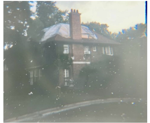
Site Photo 6, by HDC Staff, 1983: Showing damaged roof of main house at south elevation.
