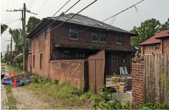
Site Photo 3, by Staff August 1, 2023: East elevation of carriage house, showing removed roof materials.
