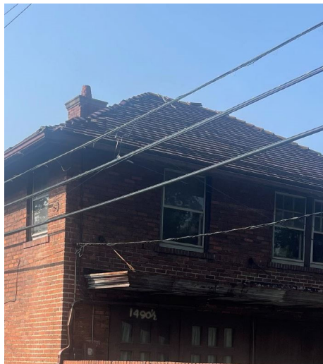
Site Photo 6, by Applicant, date unknown: Showing clay tile roof prior to removal.
