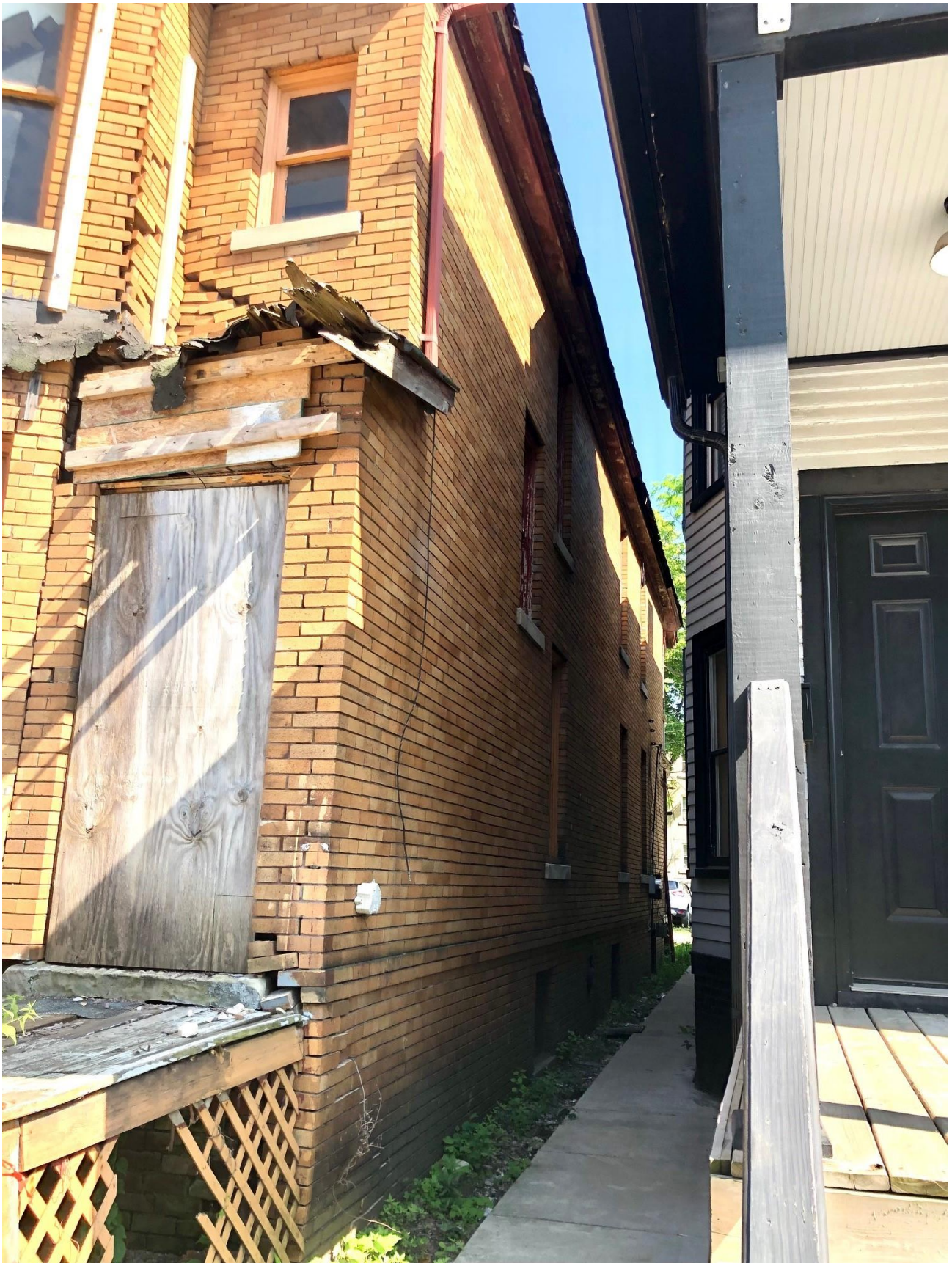
West elevation, looking south toward alley from Kercheval sidewalk. Staff photo, May 30, 2023.
