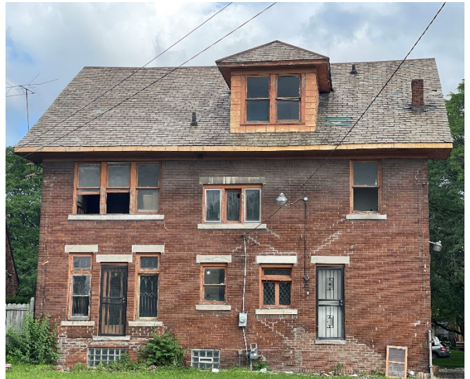
Site photo 5, by Staff, July 2023: (South) rear elevation showing missing rear steps.
