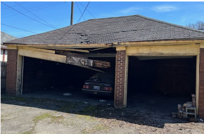
Site Photo 2, by applicant May 2023: (facing south) north elevation of garage, showing roof collapse and wood framing failure.
