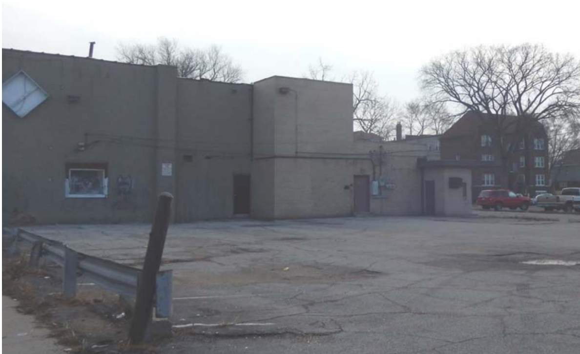
West elevation appearance in 2015 prior to rehab/establishment of west patio, staff photo. Note the lack of historic ornamentation/decorative details at this elevation.
