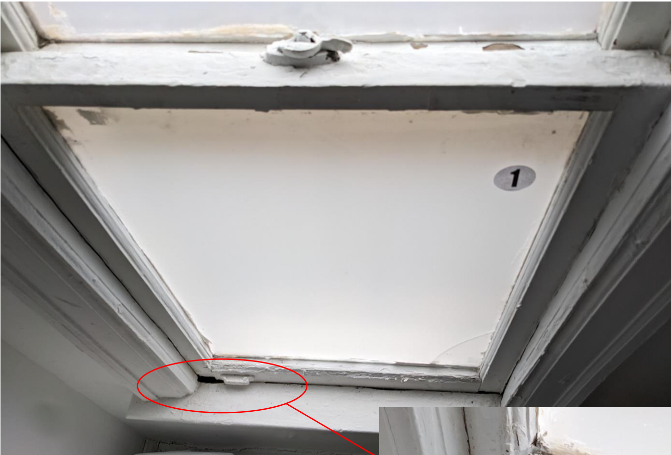
Applicant photos – Lower sash of window #1
