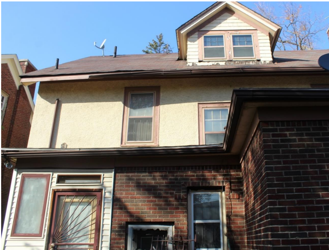
Appearance prior to the unapproved window replacement. Photo provided by applicant
