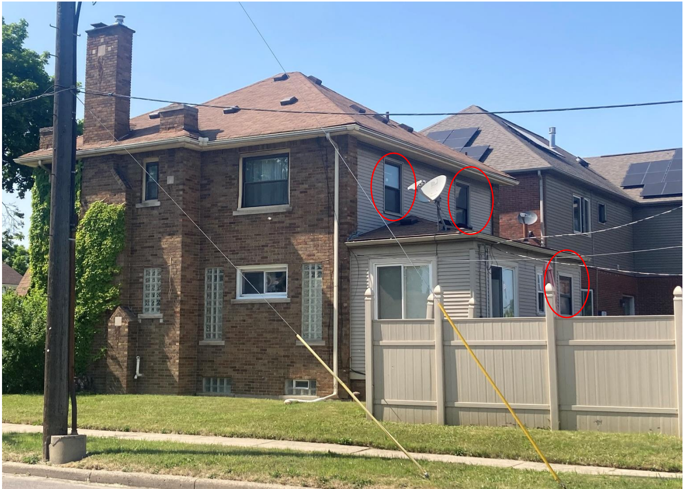
15002 Ashton, current appearance, staff photo taken 5/31/2023. The three encircled windows are proposed for replacement. Also note that the white vinyl windows were installed sometime between 2013 and 2015 before the current owner purchased the property. HDC did not approve this work.
