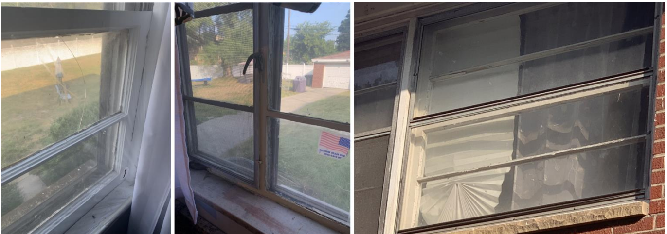
Example photos of windows proposed for replacement. Images from application; please see application for additional photos.
