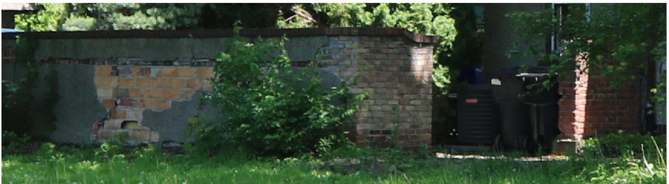
North and west faces of existing wall viewed from Iroquois. May 2023 photo by staff.
