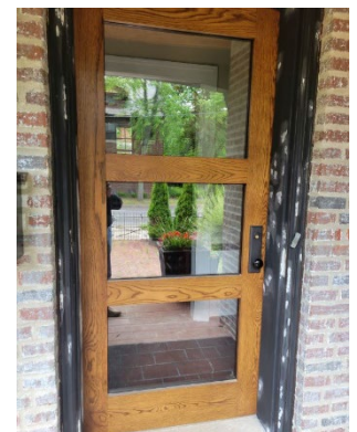
Site Photo 5, by Applicant 2023: (Southeast) front elevation, showing newly installed front door
