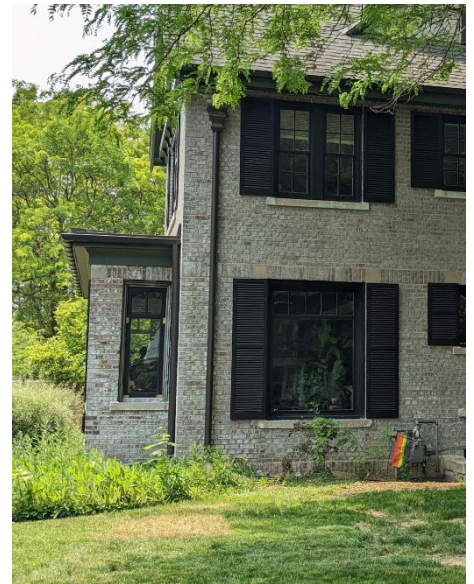
Site Photo 5, by Staff June 5, 2023: (Northeast) side elevation, detail of window #7 showing what appears to be a newly constructed wood window.
