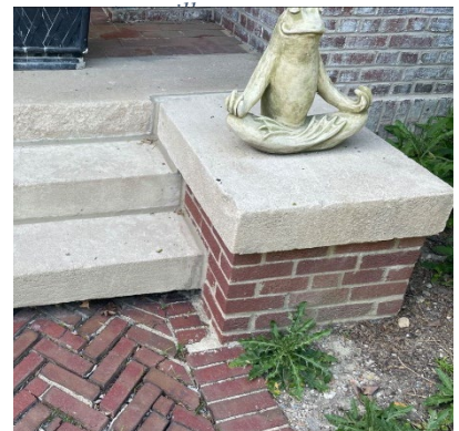
Site Photo 9, by Staff, May 24, 2023: (Southeast) front elevation, showing front porch steps and wing-walls.
