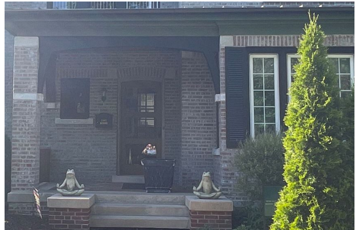
Site Photo 7, by Staff May 25, 2023: (Southeast) front elevation, showing new front door (work completed without approval).
