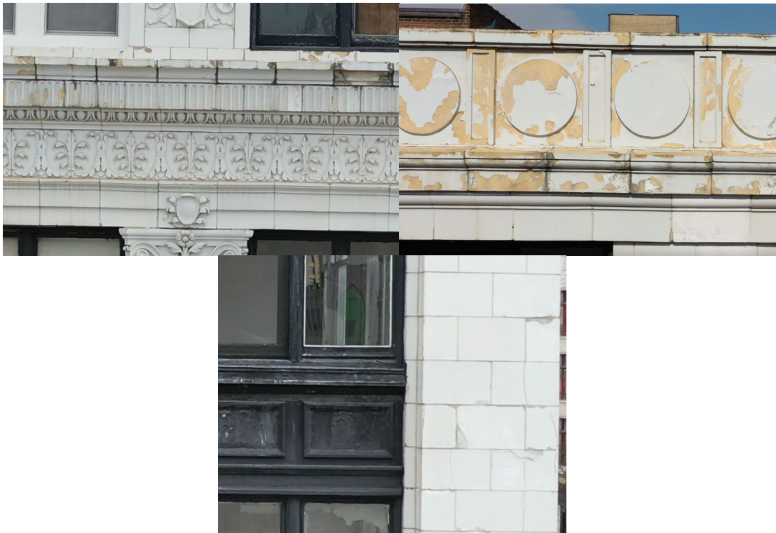
Figures 4-6: Images of existing masonry conditions provided by the applicant.
