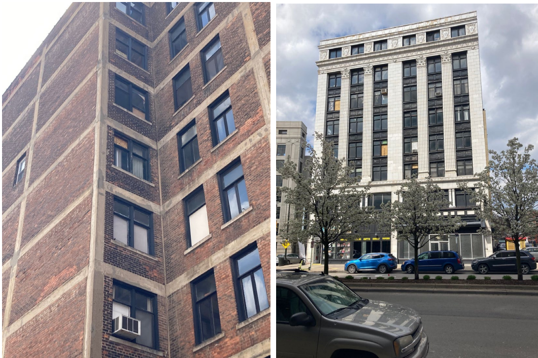
Figures 9,10: Photographs of the existing windows at the rear of the building and west façade.
