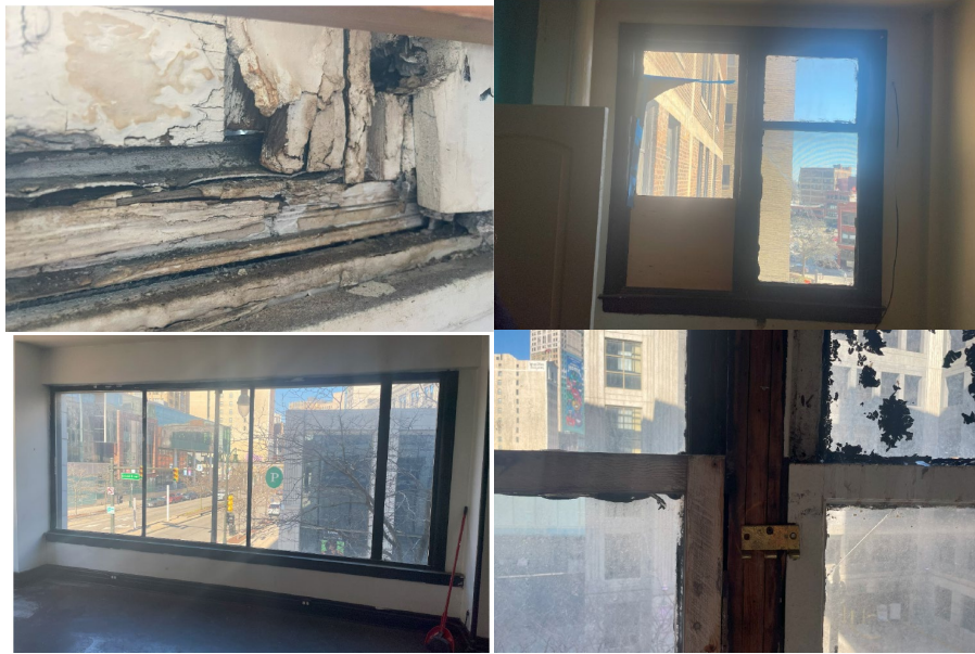
Figures 11-14: Images of existing window conditions at the interior provided by the applicant.
