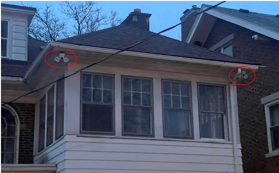
At 2027 W. Boston, two extant security light at the rear within the eaves, photo provided by applicant
