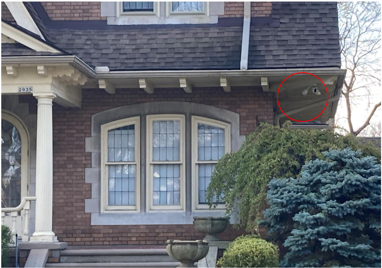
At 2035 W. Boston, detail extant security lights at the at front within the eaves, 4/23/2023 staff photos
