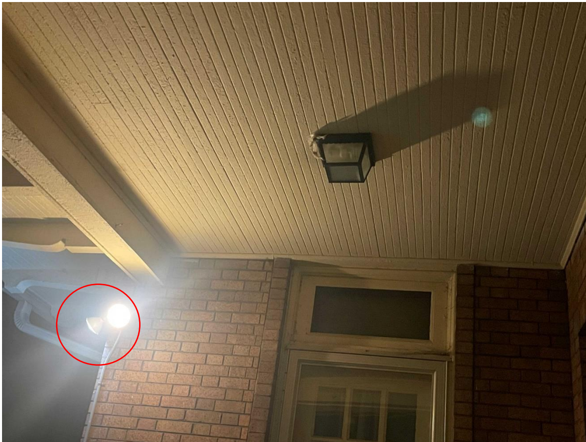
At 2035 W. Boston, one extant security light at the rear within the eaves, photo provided by applicant
