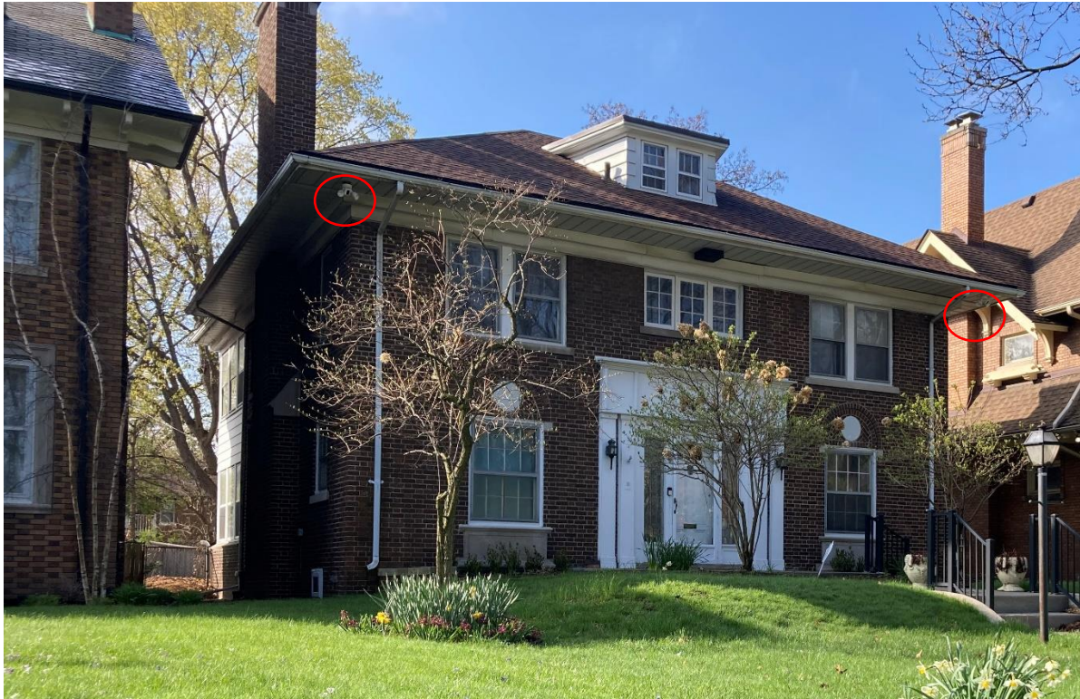
At 2027 W. Boston, two extant security lights at the at front within the eaves, 4/23/2023 staff photo
