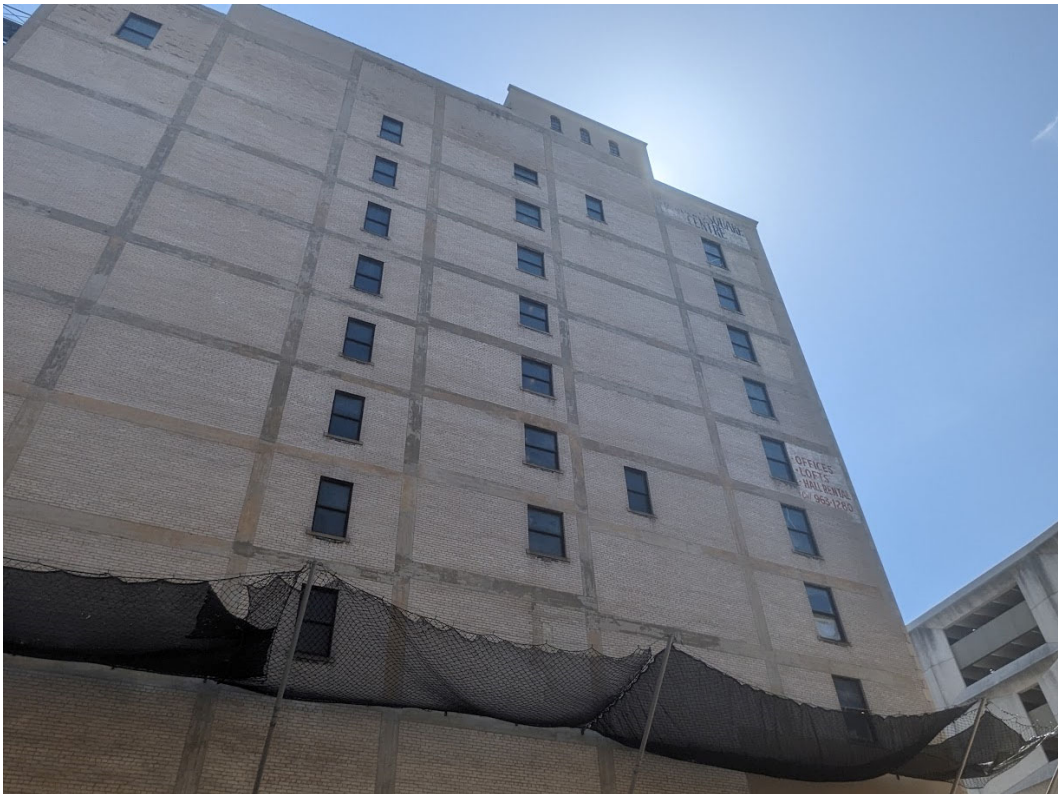
View of the west facing elevation from adjacent parking lot. Staff photo, April 19, 2023.
