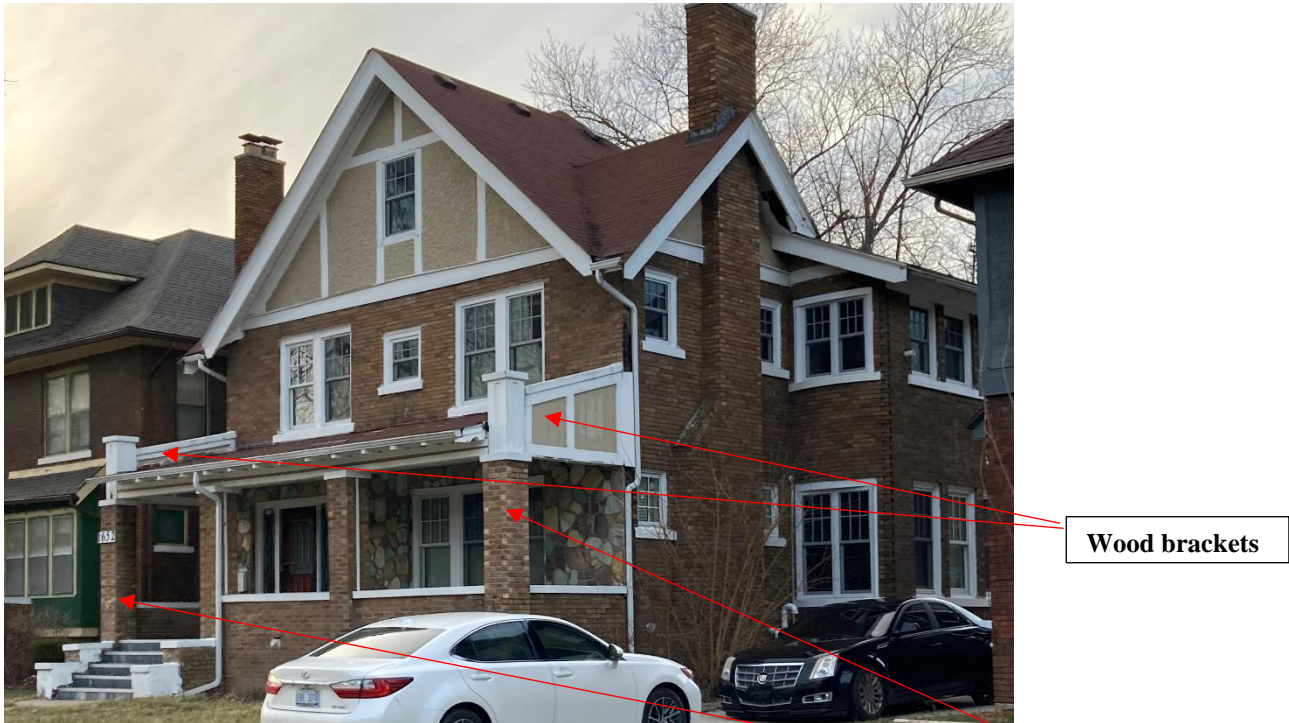
1652 Edison, staff photo showing current appearance. Note that the vinyl windows and glassblock windows were replaced in 2019 with new aluminum clad wood units and the wood has been removed from the corner columns at the front porch. However, note that the unapproved wood brackets above those columns, at the porch roof, and the slate tiles at the porch steps and floor remain.
