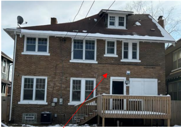
Rear of 1642 Edison, current appearance. Ghosting indicates the location of former porch (west end) removed in 2017
