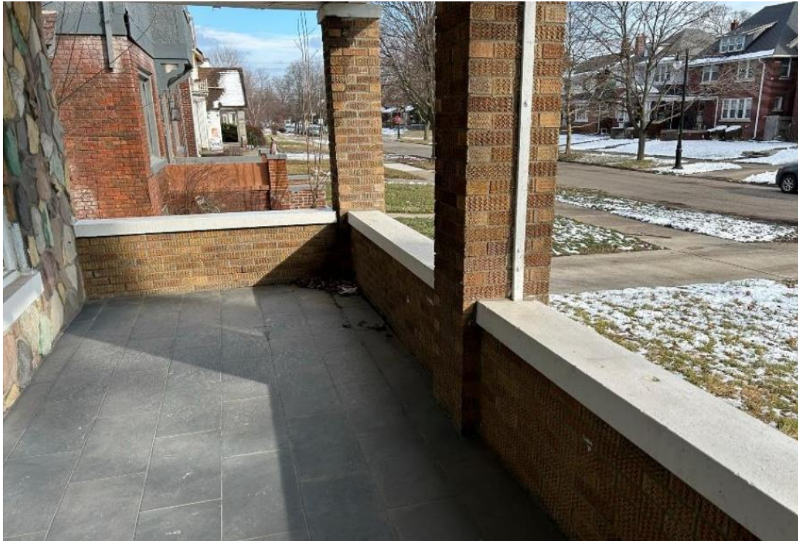
Front porch, current appearance, showing slate tiles added without HDC approval in 2017
