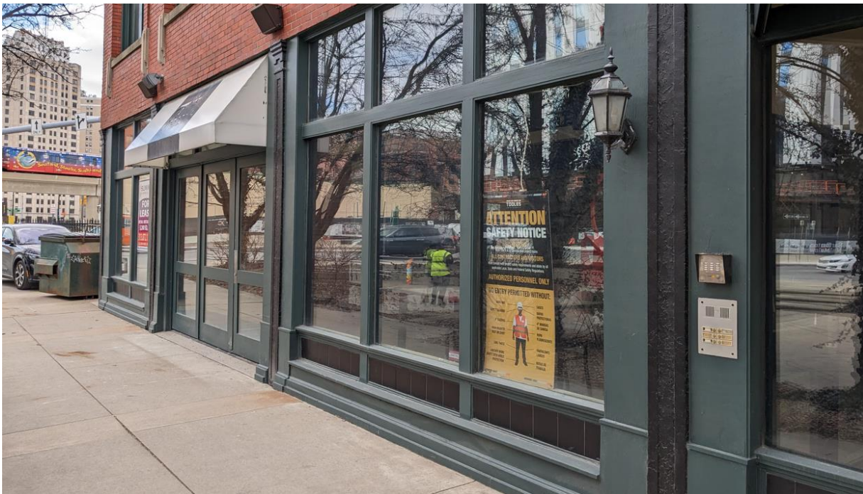
Fixed and operable storefronts at the south end of the facade. February 2023 photo by staff.
