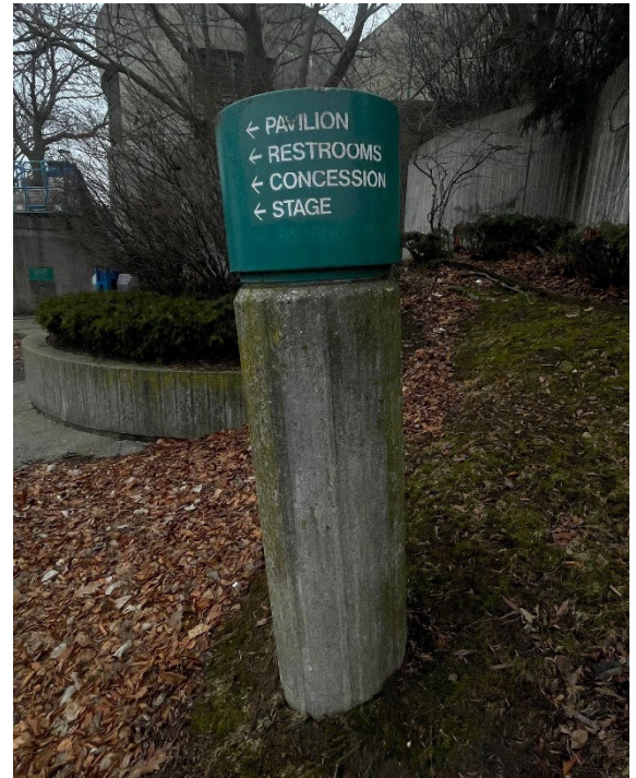
Site Photo 3, by Staff March 2, 2023: (East) near restrooms showing pylon #7 and how the striating concrete is aging like the surrounding concrete walls and complements the patterns of the surrounding landscape.
