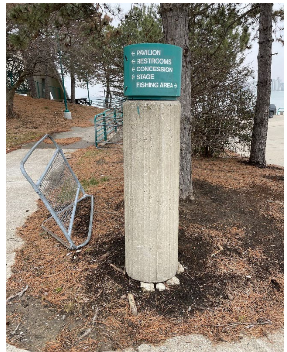
Site Photo 4, by Staff March 2, 2023: (West) Pavilion entrance showing pylon #2 and evergreens in the background that are proposed to be replaced due to disease.
