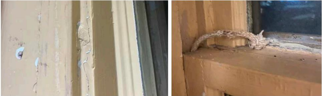
Selected examples of deterioration. Left: damaged parting bead showing overpaint. Right: Sash showing multiple layers of paint and a broken sash cord. Photos from application; cropped by staff. Please see application for additional photos and description.
