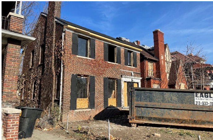
Site Photo 4, by Staff November 23, 2022: (South) front elevation, showing secure view and boarding on windows and front fascia/soffit work along the roof.
