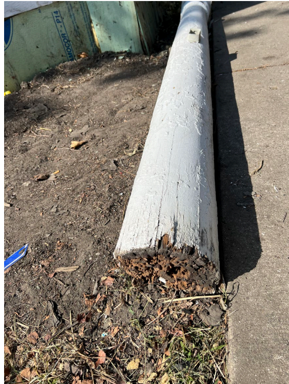
Figure 9: Image illustrating front porch column deterioration.
