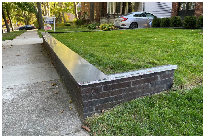
Site Photo 6, by Staff October 21, 2022: (Northeast) front elevation, showing installed retaining wall and exposed lighting under metal coping.
