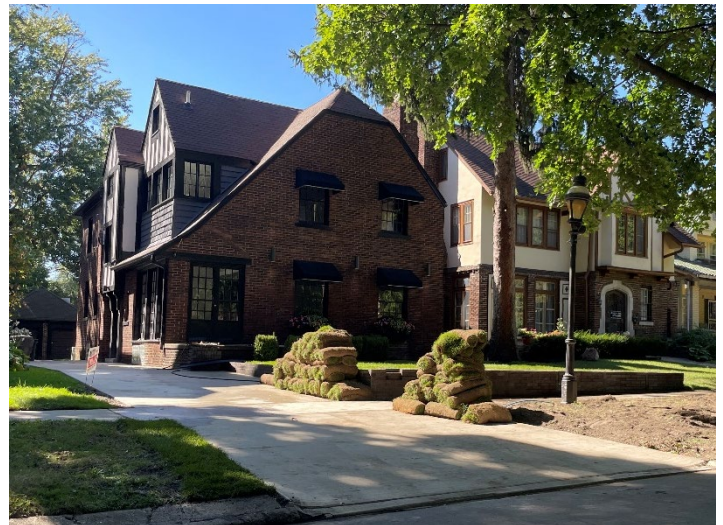
Site Photo 4, by Staff September 23, 2022: (Northeast) front elevation, showing front driveway installed, curb cut, and raised elevated front yard.
