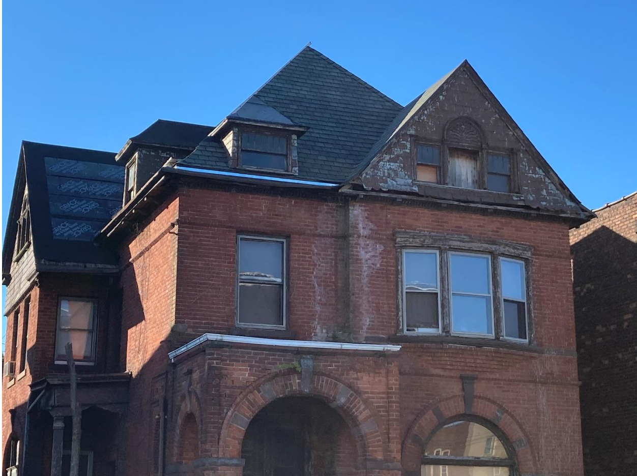
461 W. Forest, current appearance (9/30/2022 staff photos). Note that slate remains at the front and side elevation gable ends and the dormer front and side walls.
