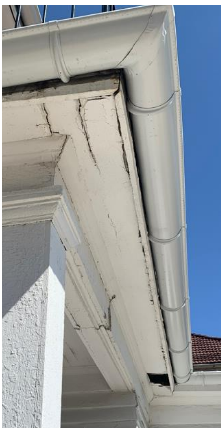
Fascia board on rear porch. Note area of missing material. Photo by applicant.
