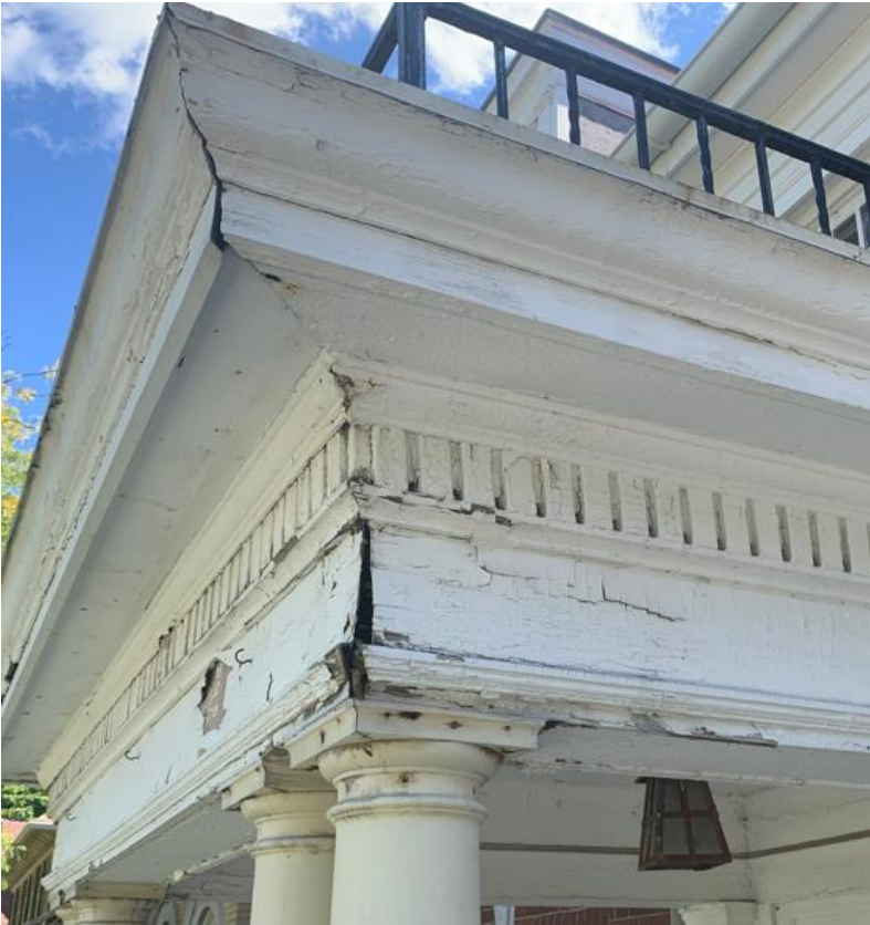
One of several deteriorated front porch areas. Photo by applicant, cropped by staff.
