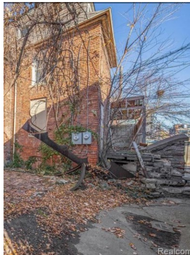
Site Photo 8, by applicant, date unknown: (South) rear, facing east elevation showing before conditions of rear covered patio. Note the presence of stone steps leading to the now boarded-up door at the rear elevation.
