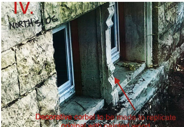
Site Photo 4, by Applicant: (North) front elevation showing before condition of front basement windows stone mullion.
