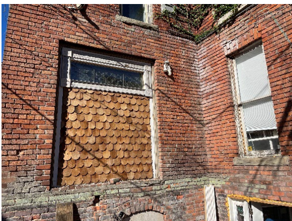
Site Photo 6, by staff, September 1, 2022 : (South) rear, east facing elevation showing location of removed doors and infill with fish-scale siding and stained glass transom from another building installed in the opening.
