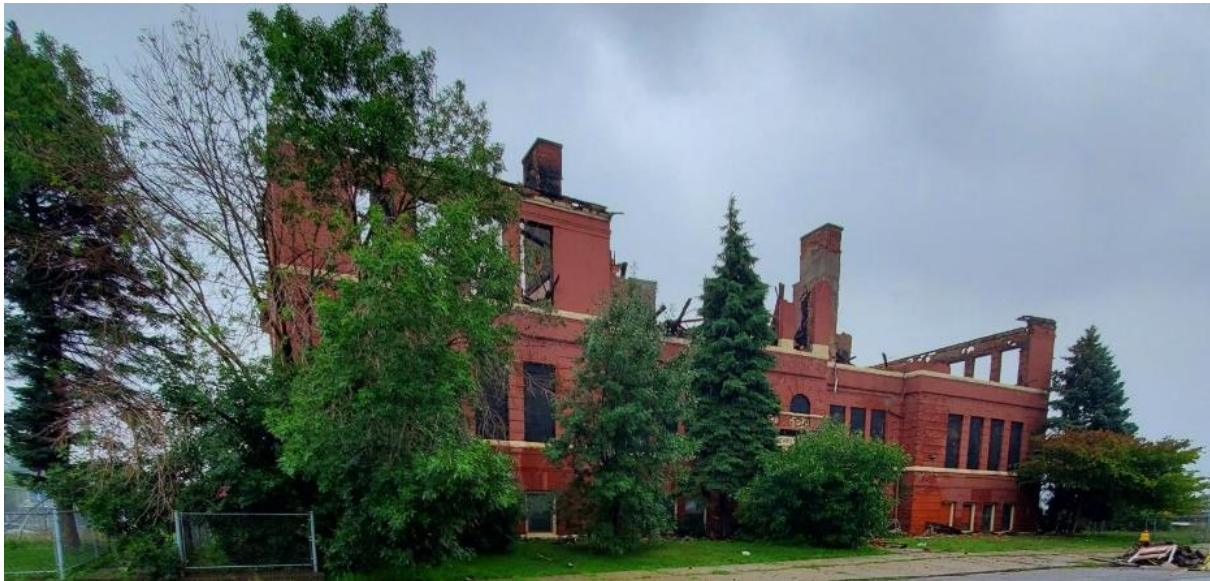
312 Waterman, BSEED staff photos showing 7/28/2022/post-fire conditions
