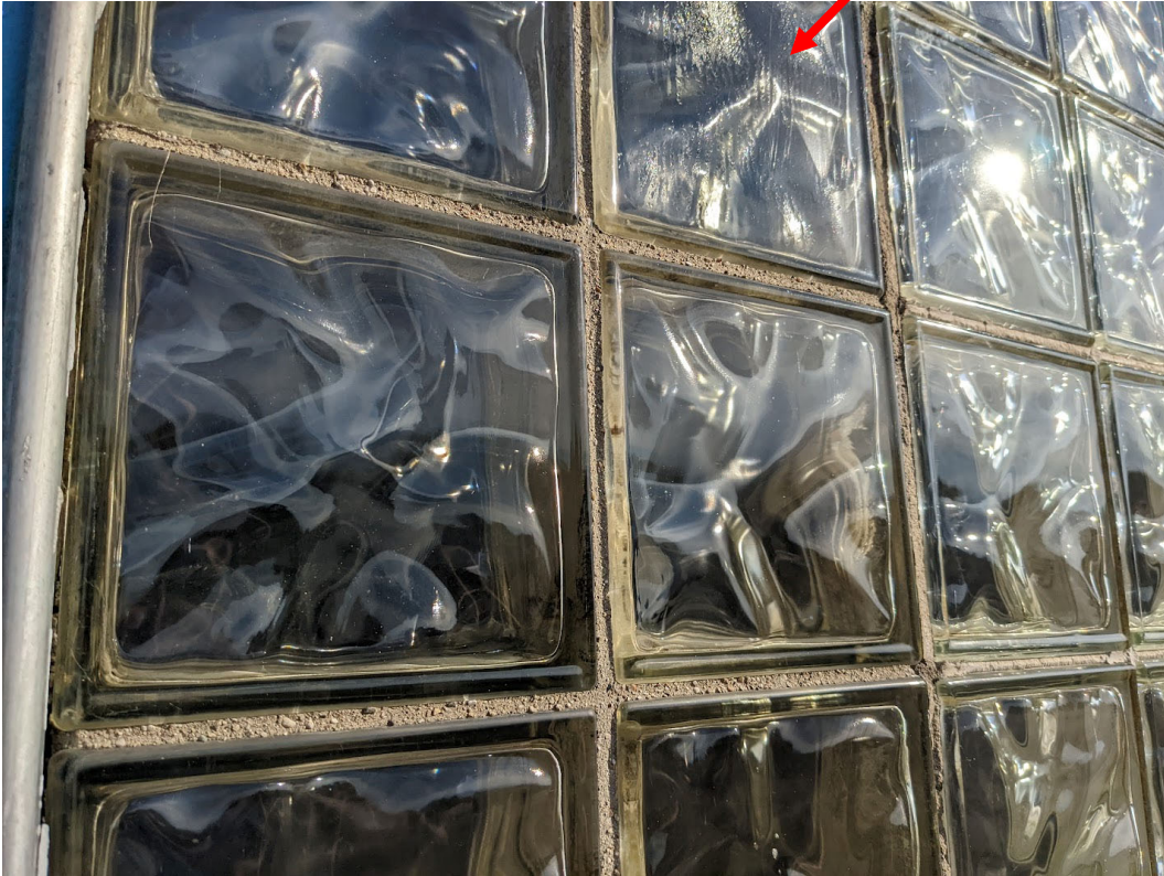
Detail view of 5021 Tireman, showing original and later glass block. One unit here (red arrow) is compromised with moisture. Staff photo, July 27, 2022.
