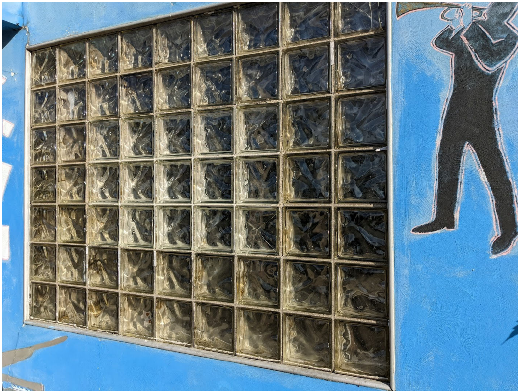
Detail view of west glass block window. Note lighter mortar joints at center. Staff photo, July 27, 2022.
