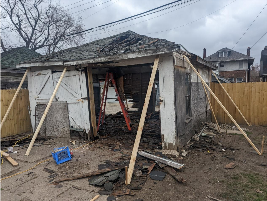
Figure 7 - Full through view (front, side, & through back) of damaged garage
