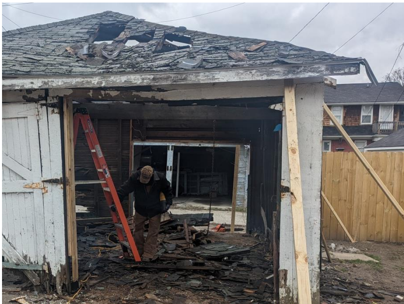
Figure 6 - See through, shored up dangerous/hazardous garage structure (note condition of roof)
