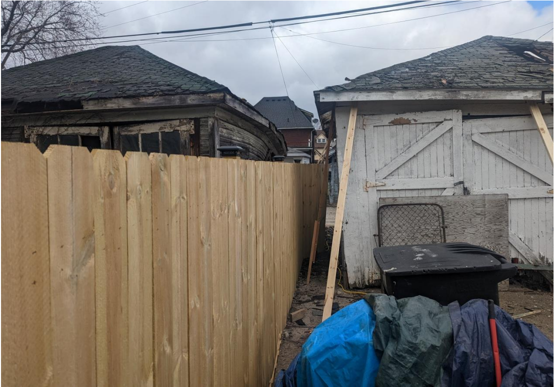
Figure 8 - Left side, near fence, of damaged garage
