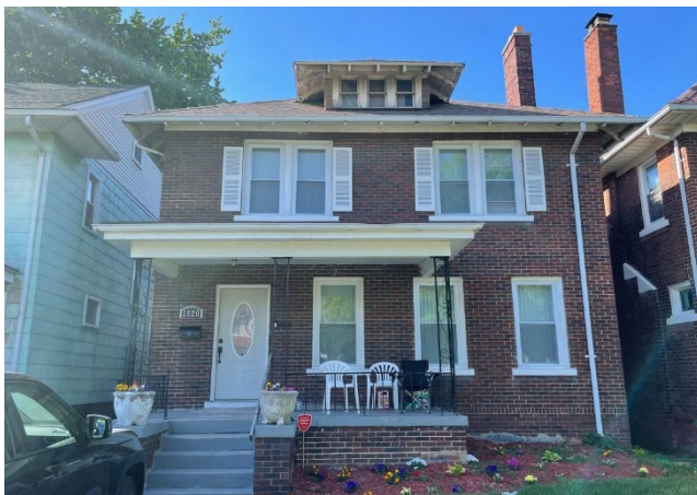
Site Photo 1, by Staff June 23, 2022: (South) Front elevation, showing original casement windows.
