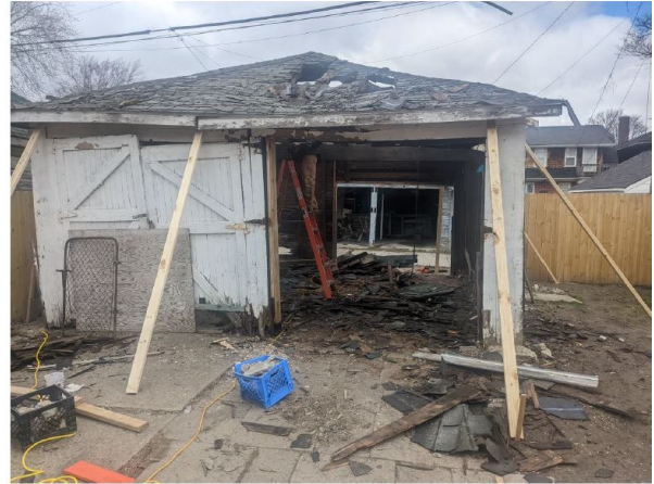
Site Photo 5, by Applicant prior to demolition of garage showing damage and bracing.
