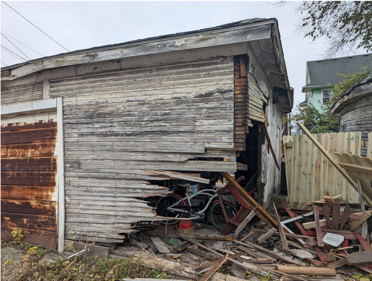
Figure 4 - Back of garage, corner hit by car
