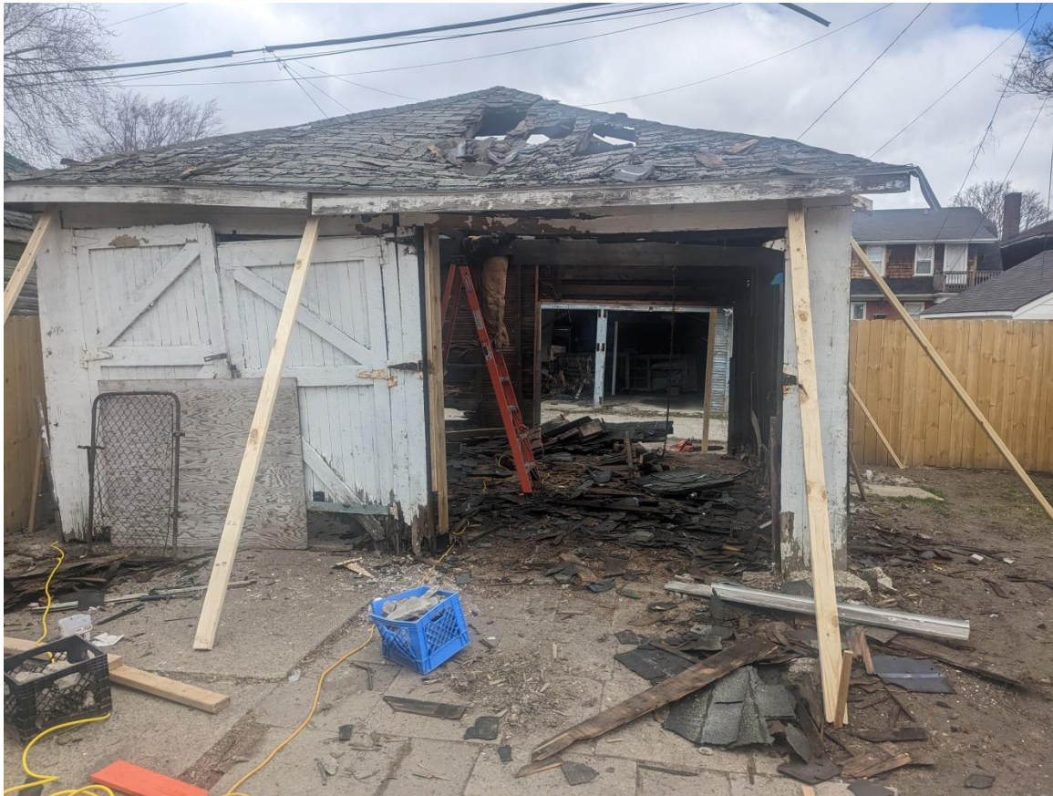
Figure 5 - Front of Damaged Garage (after having been shored up)
