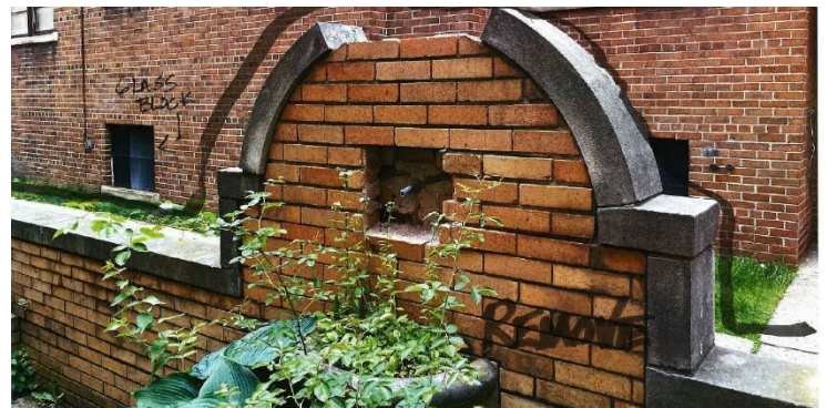
Site Photo 2 by Applicant: (South) rear elevation, showing courtyard wall fountain proposed for removal.
