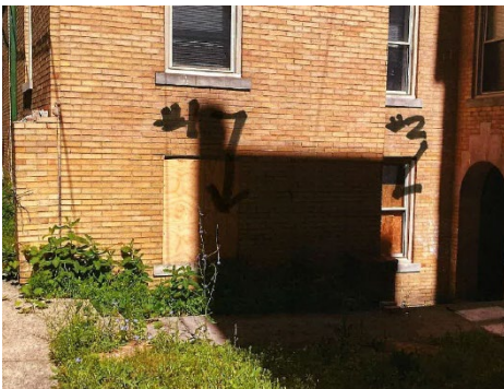
Site photo 5, by Applicant, (rear, east-facing elevation), showing proposed locations for window replacement with glass block, #1 & #2.
