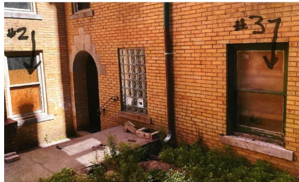
Site photo 6, by Applicant, (rear, south-facing elevation), showing proposed locations for double-hung wood window replacements with glass block, #2 & #3.
