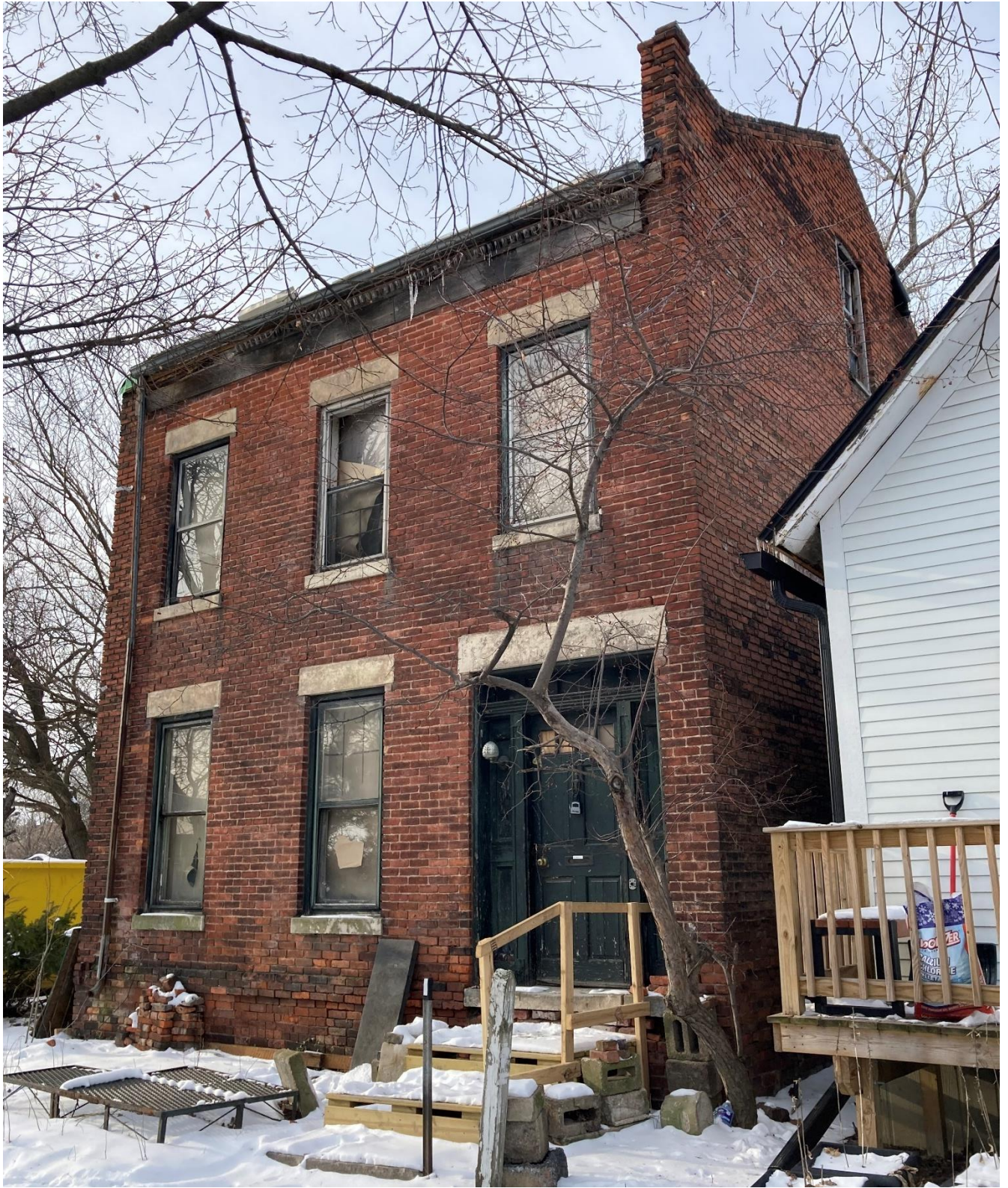
1356 Labrosse, current appearance (front elevation) showing unapproved temporary front porch deck
