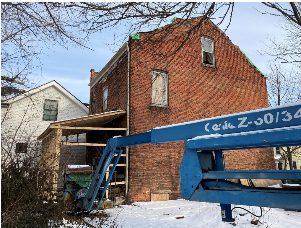
1356 Labrosse, current appearance (west elevation, showing unapproved temporary shelter at rear)
