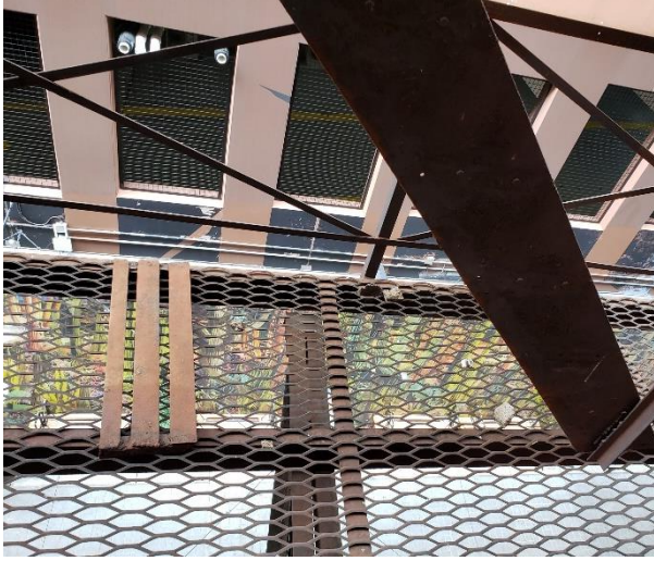
Figure 4: Fallen Stair Tread
