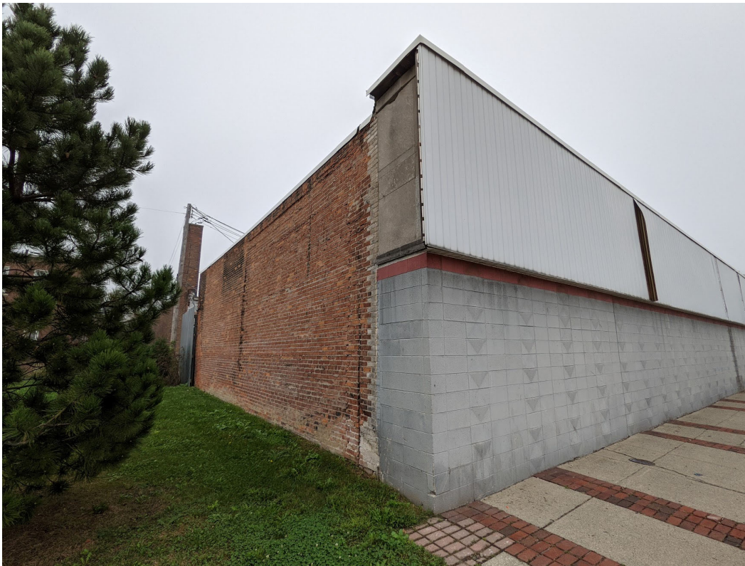
The westernmost section of historic brick buildings at 14927 East Jefferson, showing the approximately 40' of frontage subject to the Commission's jurisdiction. Note historic limestone still intact behind the incompatible white siding.
