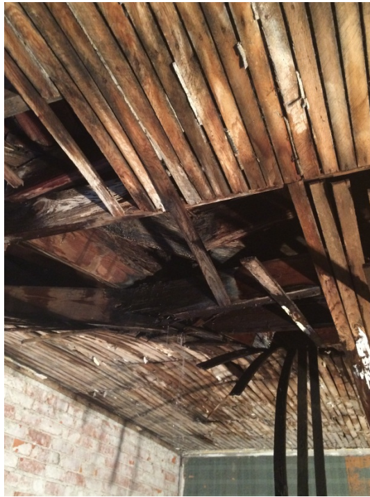
Photograph 4 – Wood roof framing failure
