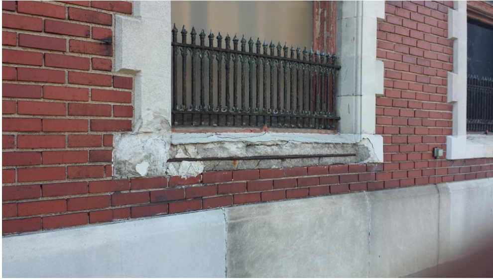
Photograph 1- Concrete window sill deterioration
