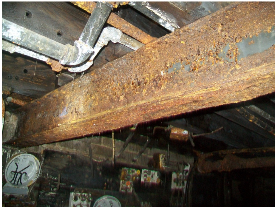
Photograph 10 – Basement. Highly corroded steel beam supporting main floor.
