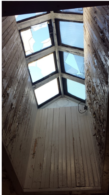
Photograph 14 – Skylight. Structural members around broken skylight exposed to the elements.
