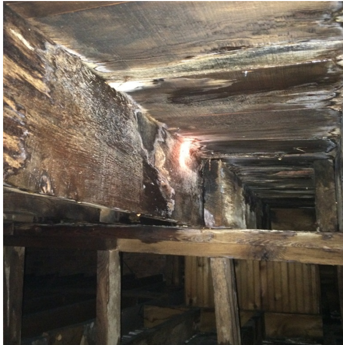
Photograph 9 – Roof framing above ceiling. Considerable water marks on wood roof framing.
