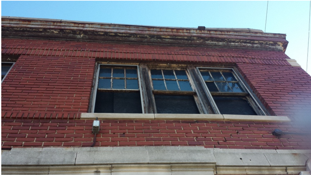
Photograph 2 – Deteriorated window lintels and metal cornice
