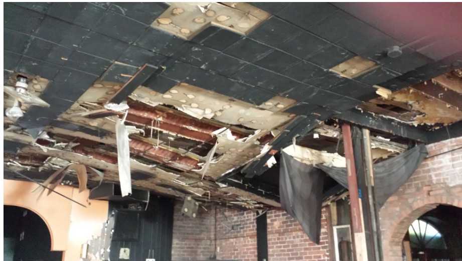
Photograph 8 – Main floor of Deck Bar. South east corner. Effects of water infiltration on ceiling.
