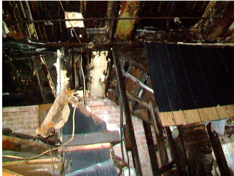
Photograph 7 – Looking at East wall of main floor of Deck Bar and stair to second floor. Rain water actively leaking through from roof. Deteriorated floor and stair framing.
