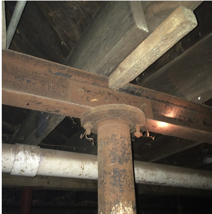
Photograph 11 – Basement – Corroded steel beam and column.
