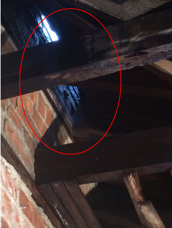
Photograph 5 – Roof at Deck Bar east wall. Large gap in roof. Structural wood joist coming out of wall bearing.
