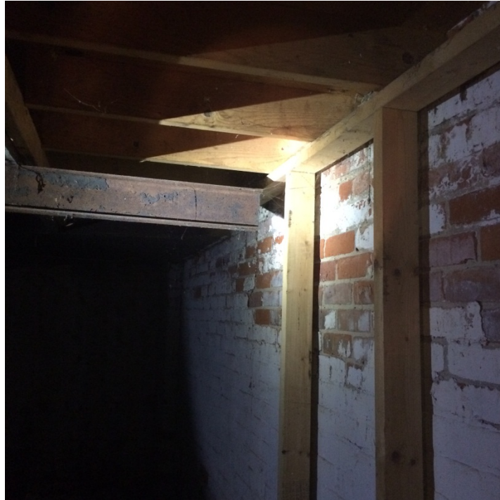
Photograph 13 – Basement – Beam cantilevered far out from support post.
