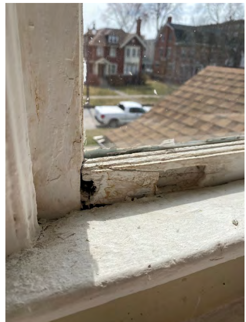
Rot at window sashes
