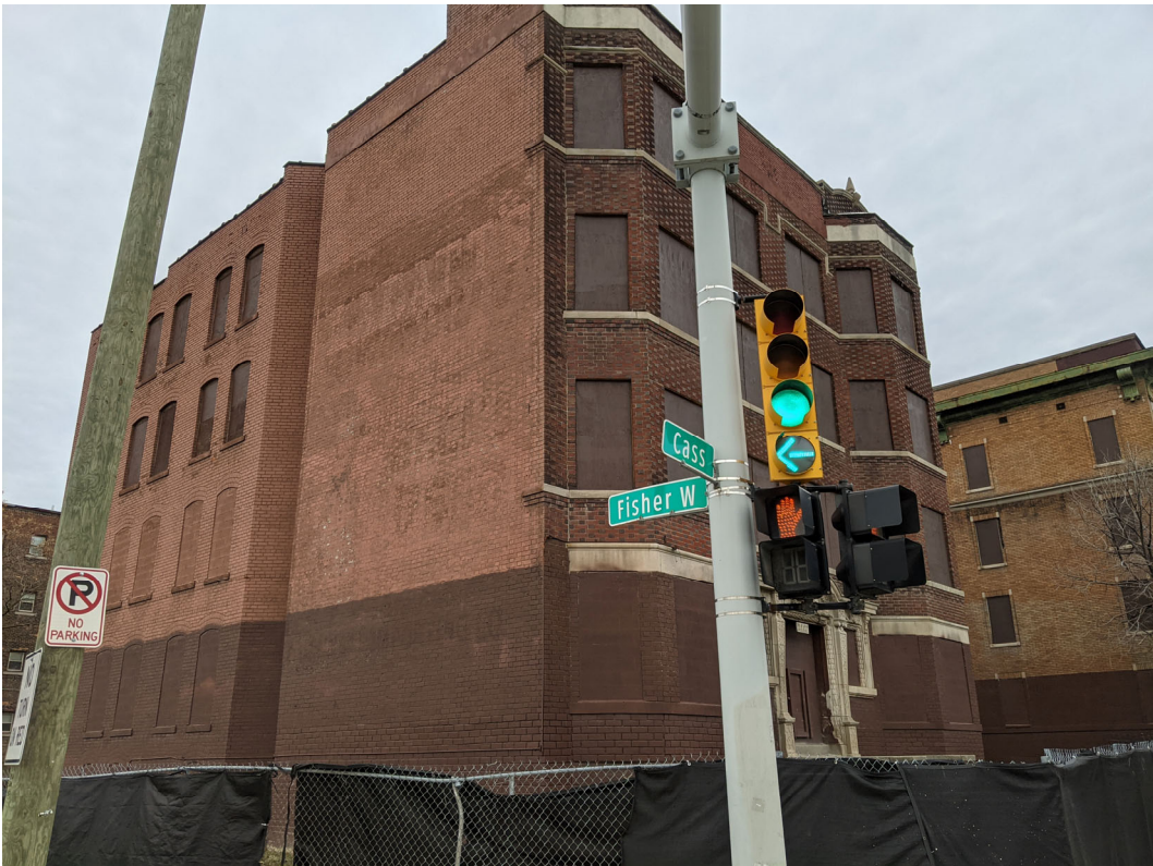
South (Fisher Service Drive) Elevation today. Note “ghost” advertisement for Labatt’s still visible. Staff photo, November 24, 2020.
