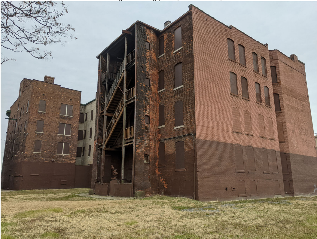
View of rear elevation, looking northeast. Note exterior stairs. Staff photo, November 24, 2020.
