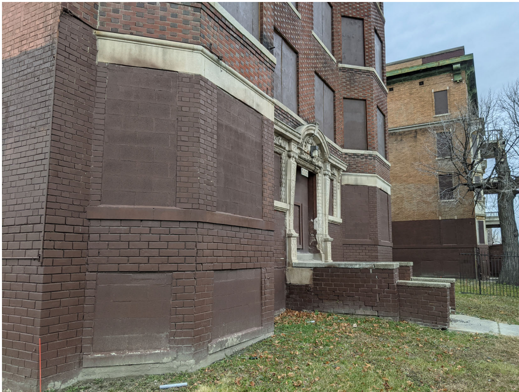
Detail view of Hotel Ansonia first story, with the Atlanta (2467 Cass) beyond, representing the eastern extents of the Cass-Henry Historic District. Note extent of brown paint. Staff photo, November 24, 2020.
