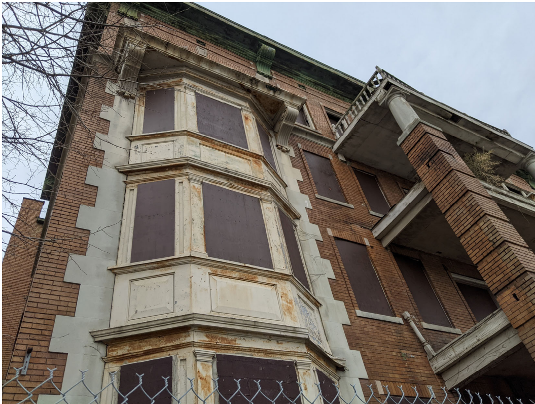
Detail view showing conditions at the Cass (primary) facade. Staff photo, November 24, 2020.
