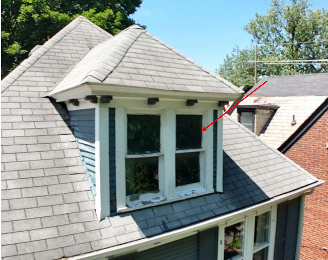
Windows at front dormer proposed for replacement (red arrow), photo by applicant.
