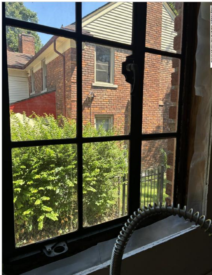
Interior photo of the north-side kitchen window. It is a centered casement window with fixed windows surrounding it and it appears to staff that a crank may be missing. An awning window is proposed to be installed. (Applicant photo)
