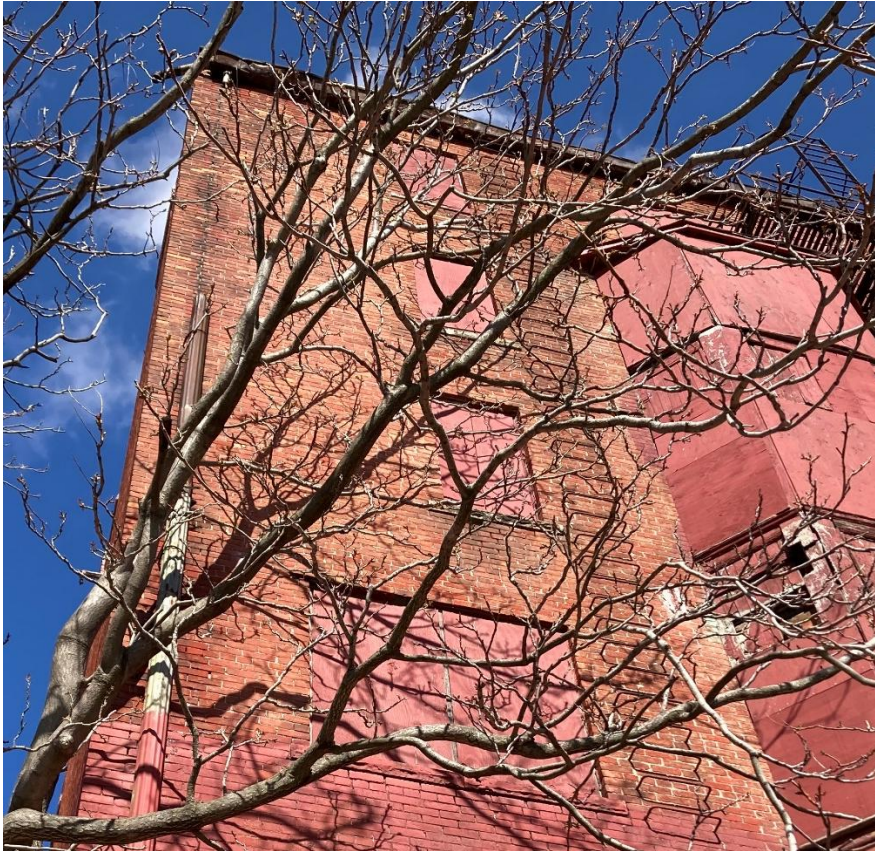
Existing gutter and downspout on the west end of the building. The gutter looks like a simple box gutter but the downspout is round, fluted metal. This end of the building is secondary and probably would not have been seen well historically because of neighboring buildings, but currently the building stands quite alone and can be viewed from all sides. (Detail, staff photo, 2026)
