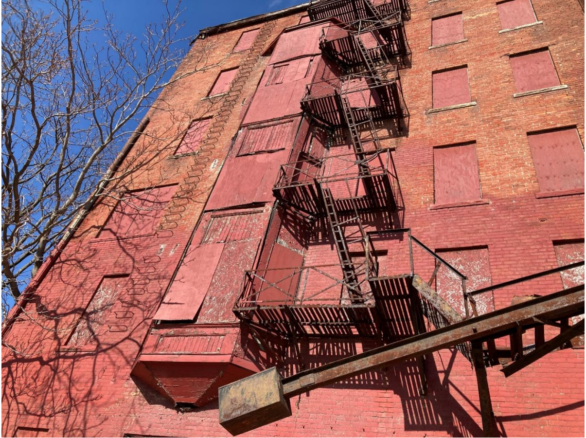
West end of the building. Staff is not certain whether these counterbalanced stair fire escapes were also installed in 1940, but the design of the balconies, railings, and counterweight are all similar to the fire escapes on the east end. The west end's stacked bay windows are also visible in this photo. (Staff photo, April 2026)
