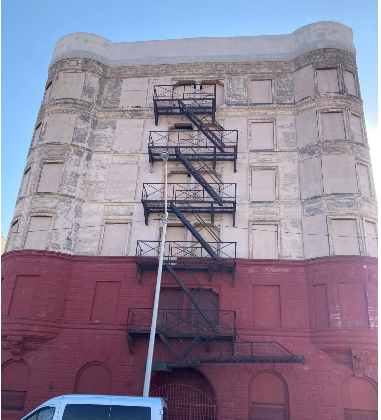
The counterbalanced fire escape stairs on the Park Avenue (east) end of the building. The “Xs” on the balcony railings are not visible in the 1970s photo, but the size of the balconies, the placement of the attachments, the angle of the stairs, the counterweight, and the railing on the lowest section of stair that would pivot to the sidewalk all match the 1970s photo. (Staff photo, April 2026)
