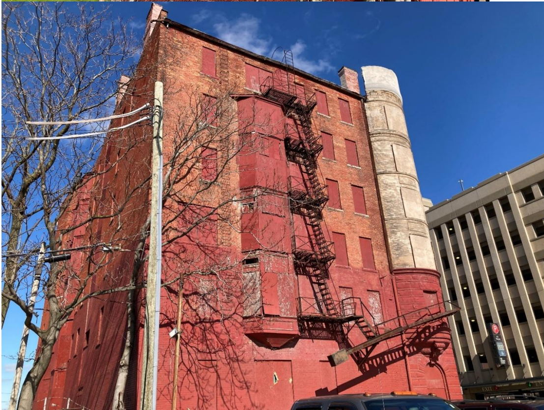
The north side (top) and west end of 100 Temple. The multi-story bay windows, covered in painted plywood, are visible on both and are proposed to be removed, reframed, and boarded and then finished at a later time. (Staff photo, April 2026)
