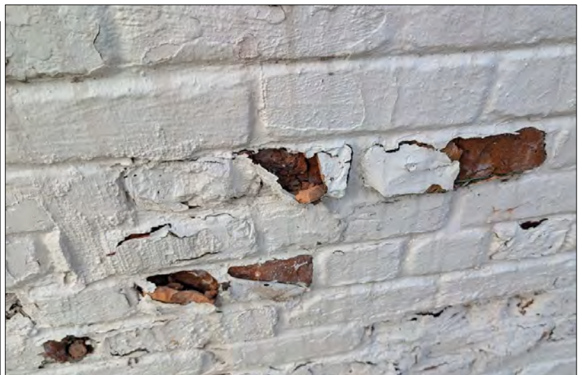
Historic-age Detroit building exhibiting paint slowly destroying the brick wall through spalling and moisture retention.
