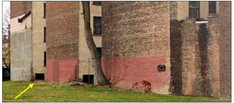
View of previous retaining wall/fence condition - it appears that the fence was no longer in place at this rear location. Google Streetview, 11/2024.
