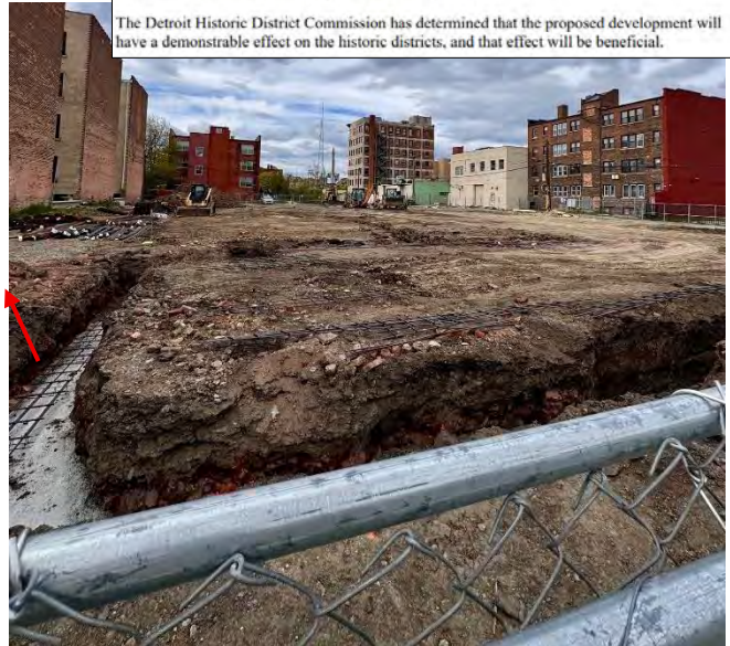
Looking north from MLK Jr. Blvd. sidewalk. East walls of 470 MLK Jr. Blvd at far left.
