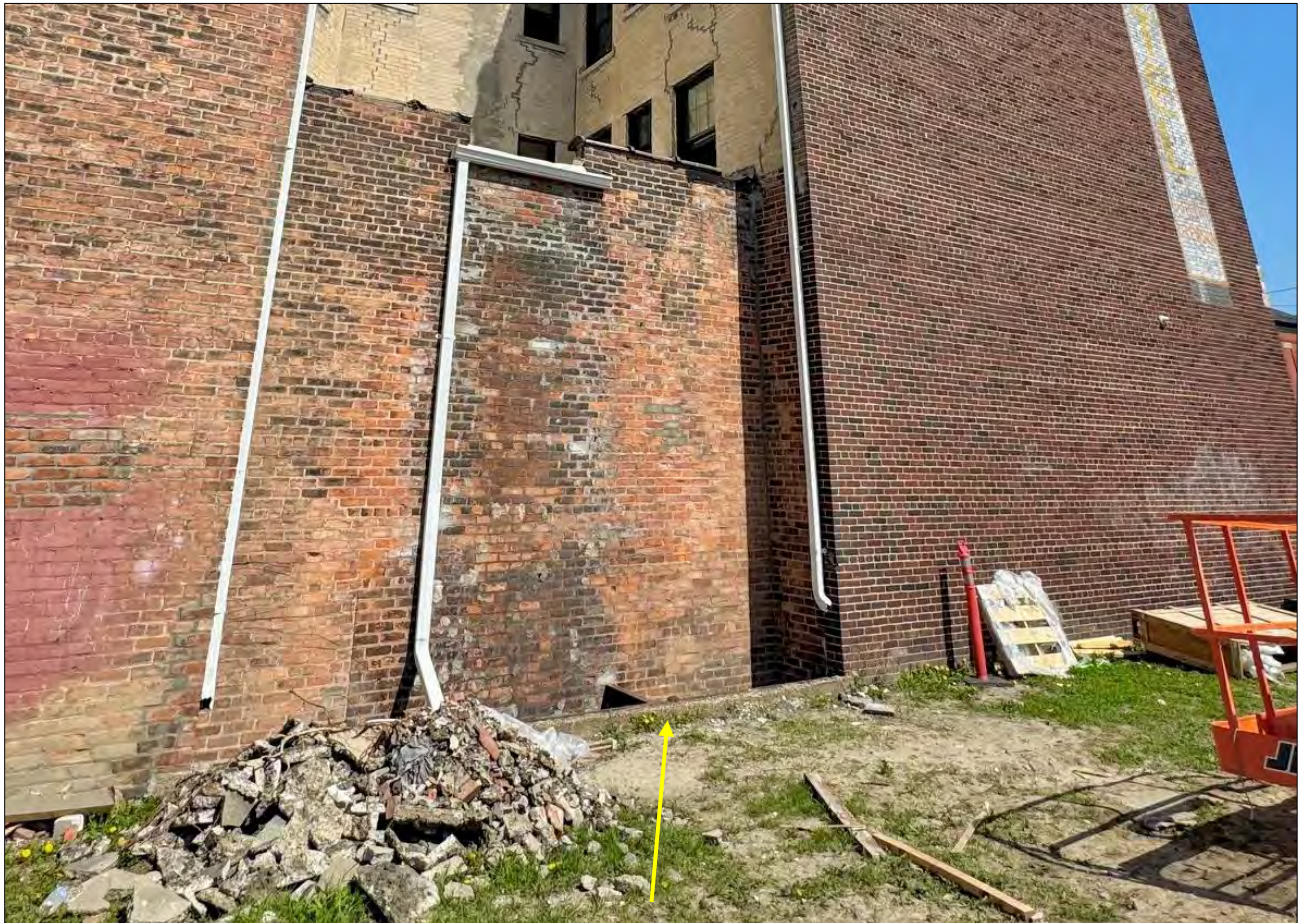
At this historic enclosure spanning the front two bays, the historic age concrete retaining wall/foundation remained in place during staff's first site visit. Staff photo, 04/22/2026.
