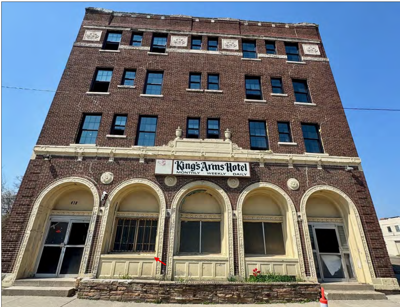
Staff photo, taken on 04/22/2026, shows the replacement of the 2 nd – 4 th floor windows is complete. The remaining intact historic-age double casement at the first floor is clearly visible.
